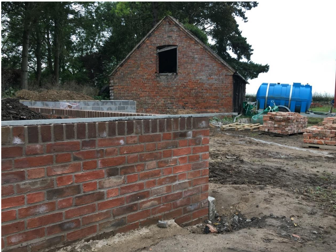
Watergate Blend brick used to boundary wall on Raby Estate set against existing farm outbuilding
