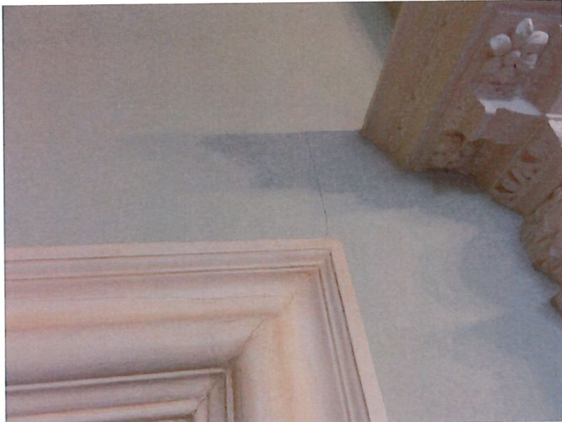
Photo 13 – Crack adjacent door head
