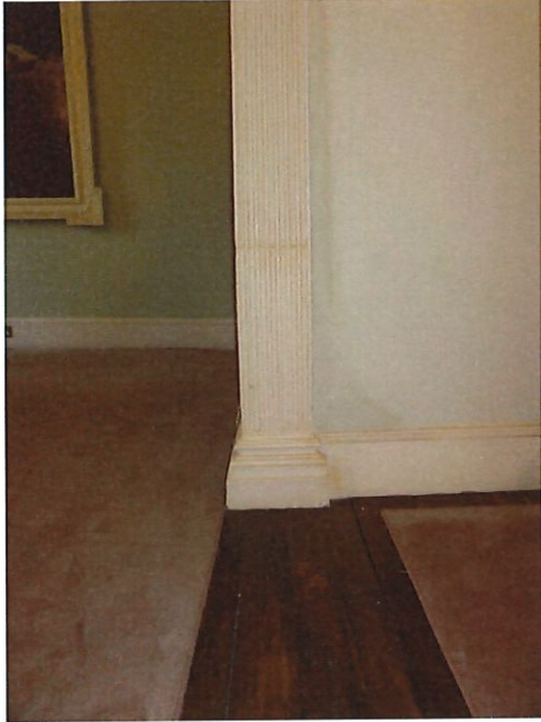
Photo 11 – Floor dropped and slight rotation of wall/pier
