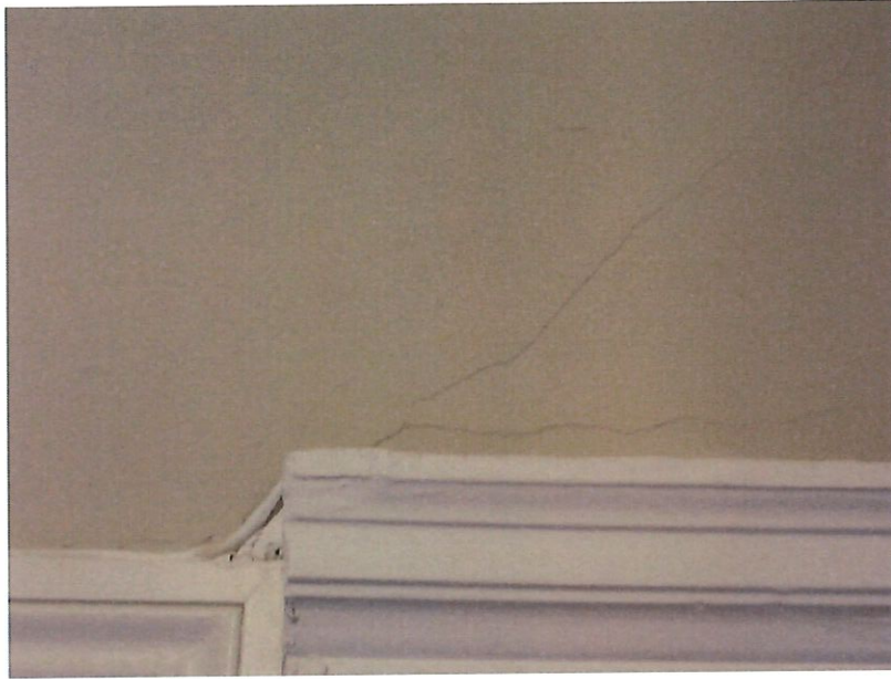
Photo 17 – Diagonal crack over architrave
