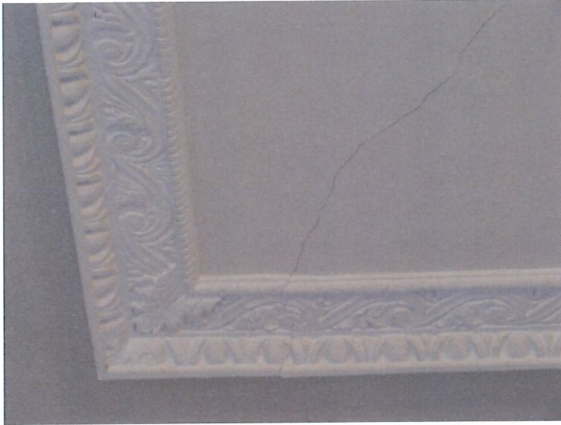
Photo 19 – Ceiling cracks over small dining room.
