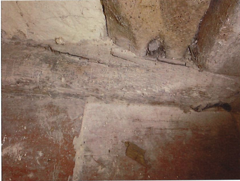
Photo 3 – Compression of decayed timber
