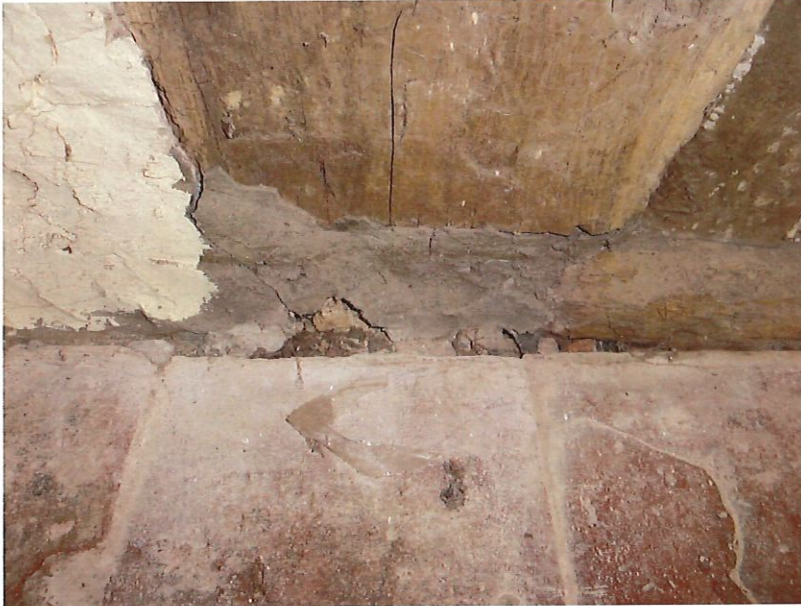
Photo 7 – Historic repair to sill
