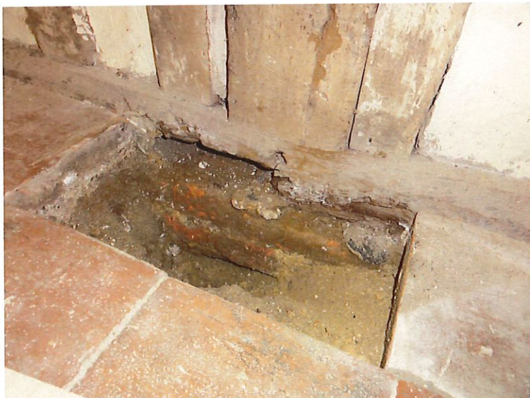
Photo 2 – Decay of sill plate
