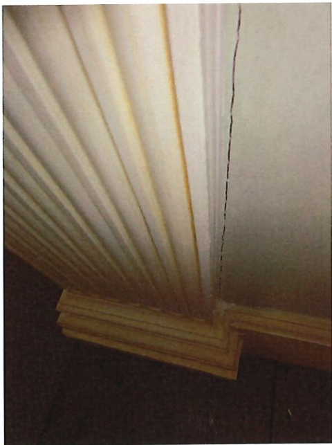
Photo 12 – Crack (vertical) adjacent decorative pier
