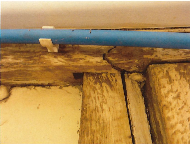
Photo 6 – Fractured header beam
