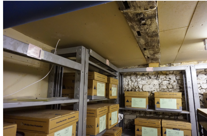
Fig. 8 - Store room showing bressumer with empty mortises
