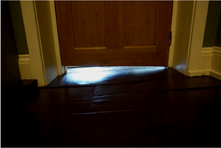
Fig. 10 - Detail showing deflection under ground floor door
