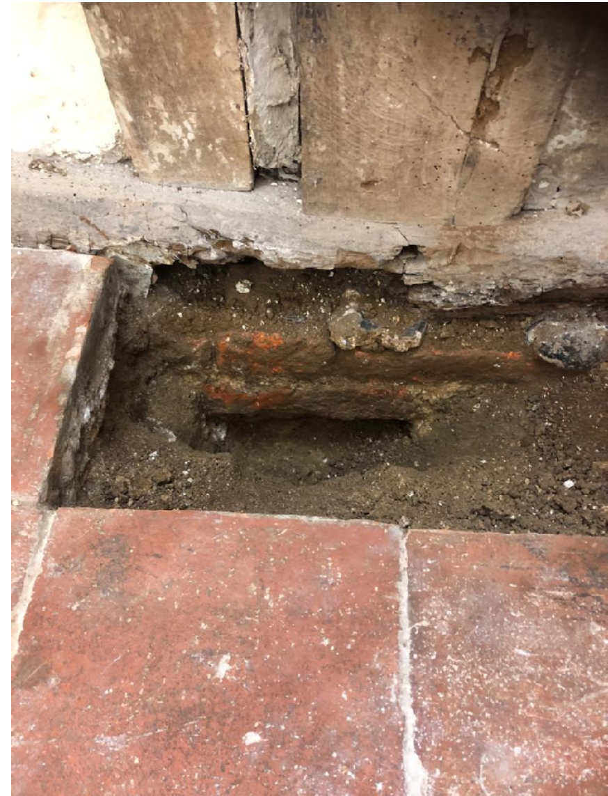
Fig. 9 - Detailed view of failed sole plate and brick plinth
