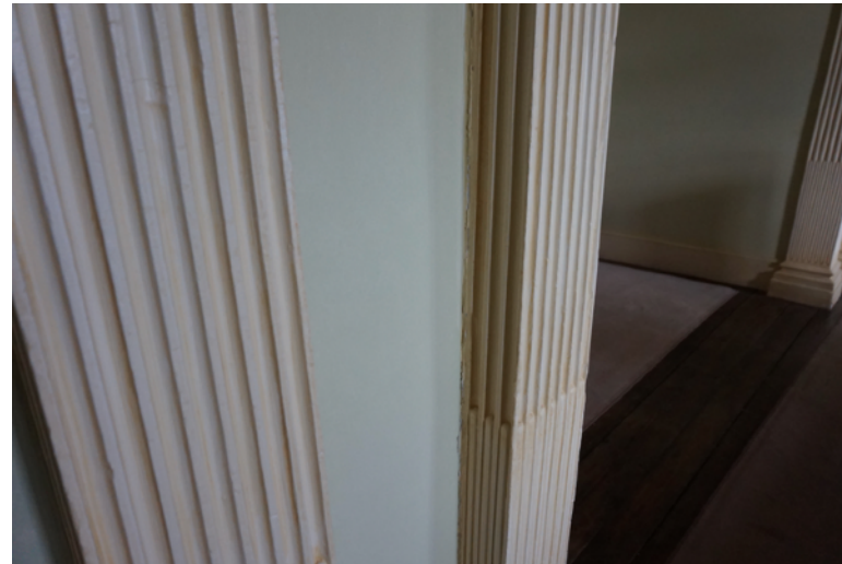
Fig. 12 - Detail of cracking to pilaster
