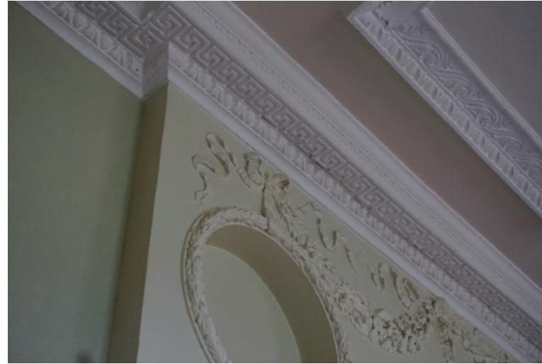
Fig. 11 - Cracking to 18th century plasterwork
