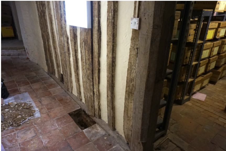
Fig. 7 - Timber framed wall, showing sole plate predominately below floor level.
