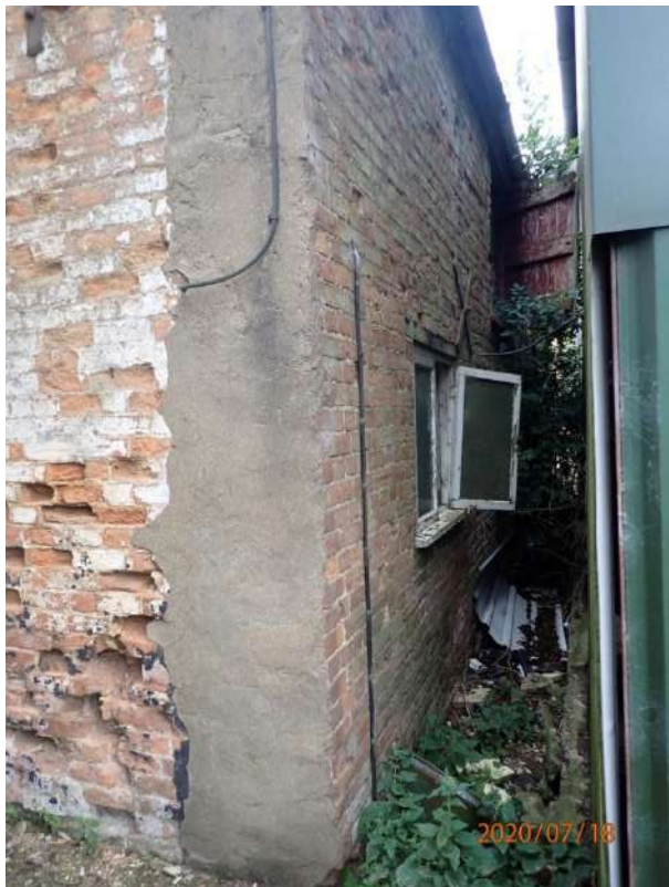
Plate 173: View of the East Elevation of the East Range, from the south
