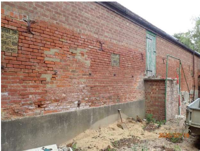
Plate 179: View of the East Elevation of the East Range, from the south-east
