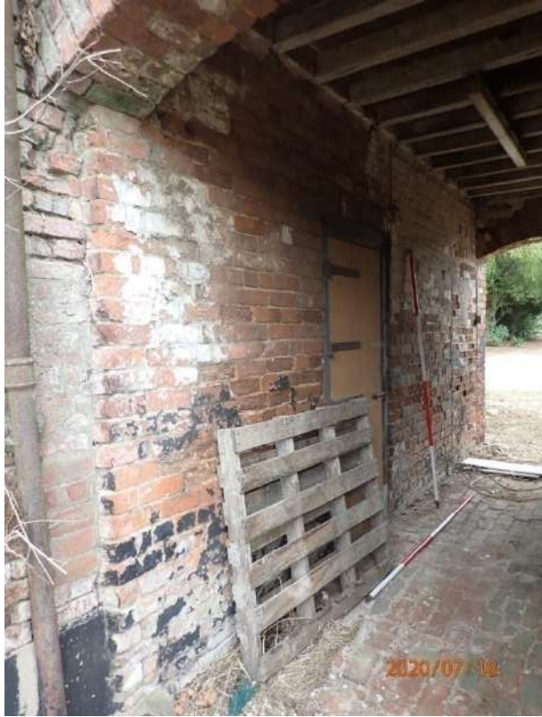
Plate 191: View of the north wall of the northern tunnel within the East Range, from the west
