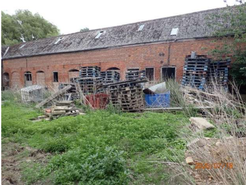
Plate 193: General view of the West Elevation of the East Range, from the west
