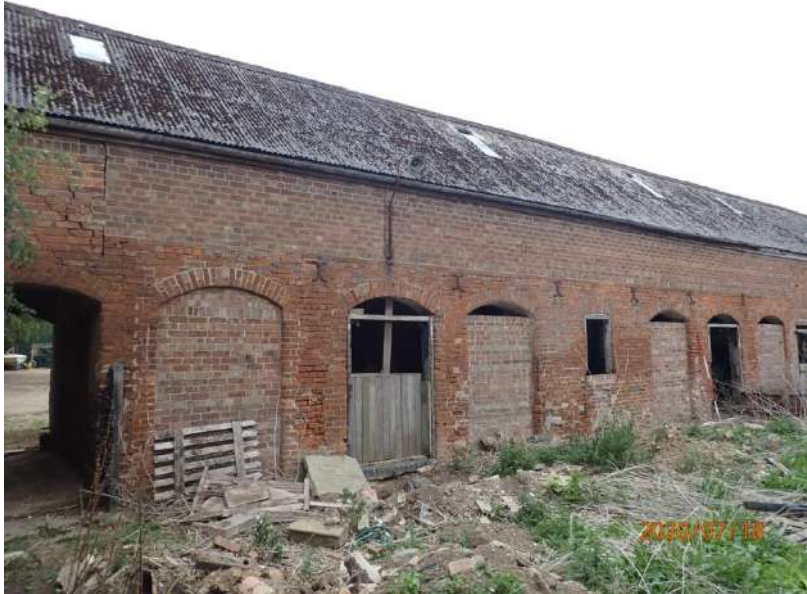
Plate 195: View of the West Elevation of the East Range, from the north-west
