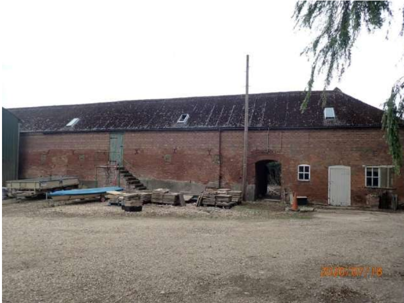
Plate 176: View of the East Elevation of the East Range, from the east
