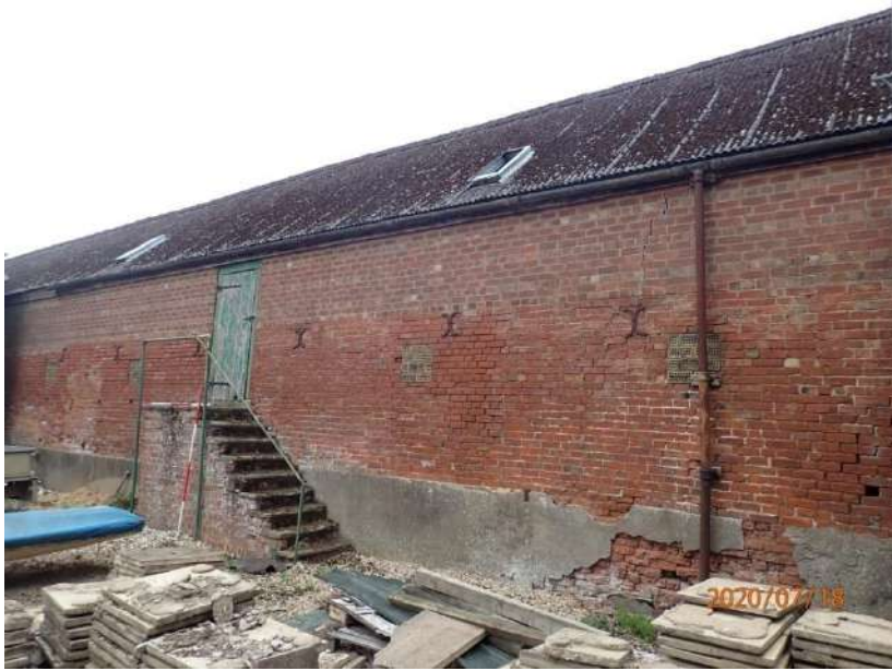
Plate 180: View of the East Elevation of the East Range, from the north-east
