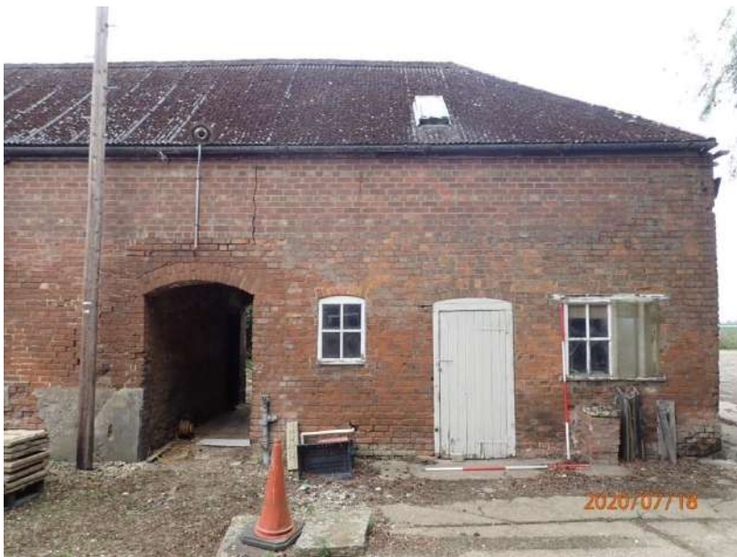
Plate 181: View of the East Elevation of the East Range, from the east
