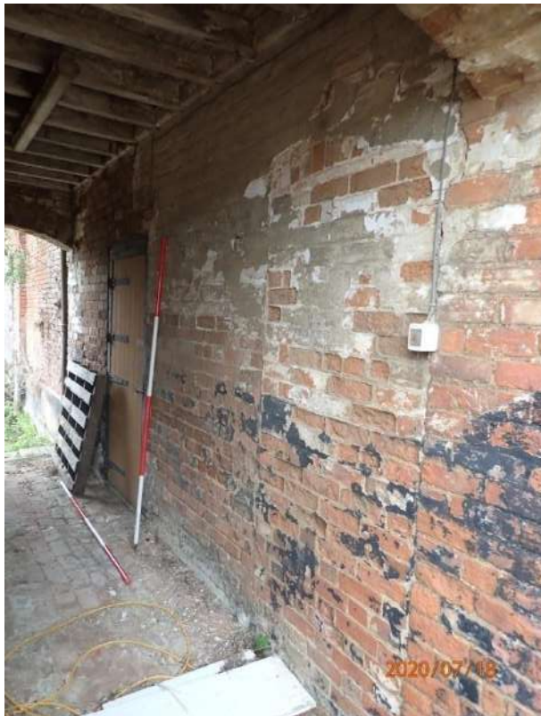
Plate 190: View of the north wall of the northern tunnel within the East Range, from the east
