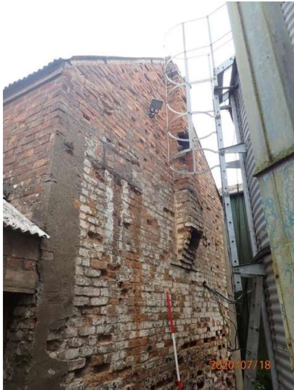
Plate 169: View of the South Elevation of the East Range, from the west
