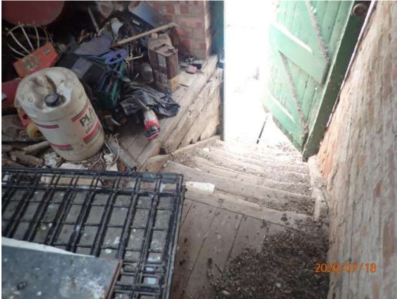
Plate 338: View of the stairwell, down to the exterior of the building, from the west
