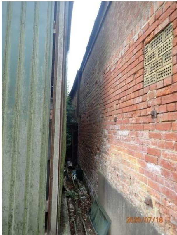
Plate 175: View of the East Elevation of the East Range, from the north
