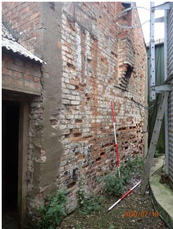
Plate 168: View of the South Elevation of the East Range, from the west
