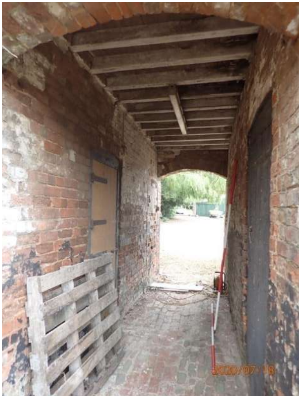
Plate 188: General view of the interior of the northern tunnel within the East Range, from the west
