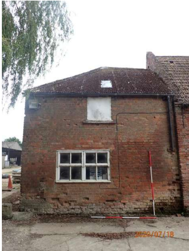
Plate 166: View of the North Elevation of the East Range, from the north
