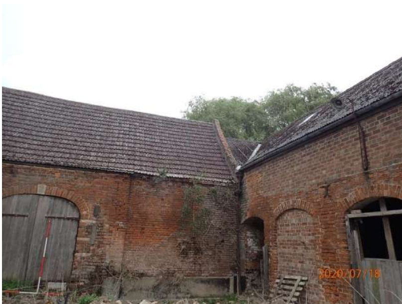
Plate 194: View of the West Elevation of the East Range, from the south
