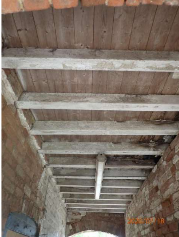
Plate 185: View of the interior of the northern tunnel within the East Range, from the west
