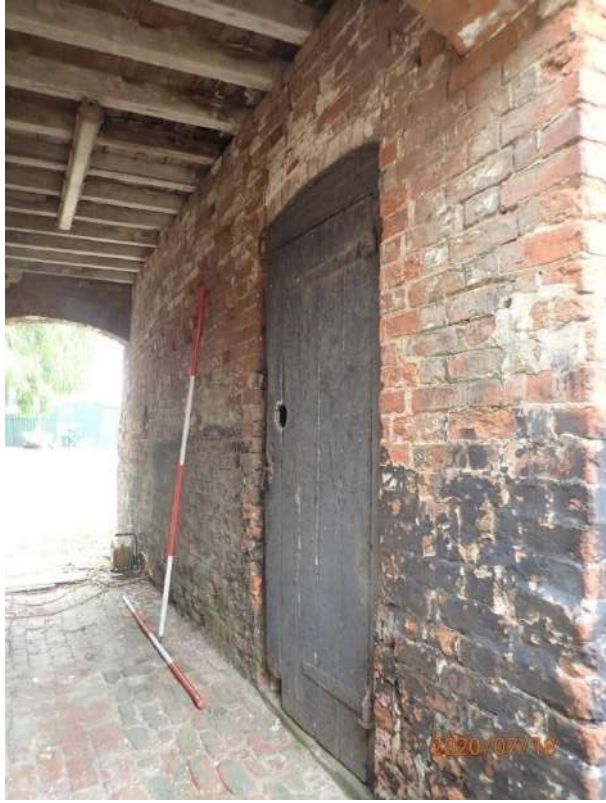
Plate 189: View of the south wall of the northern tunnel within the East Range, from the west
