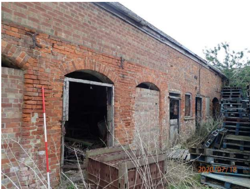
Plate 198: View of the West Elevation of the East Range, from the north-west
