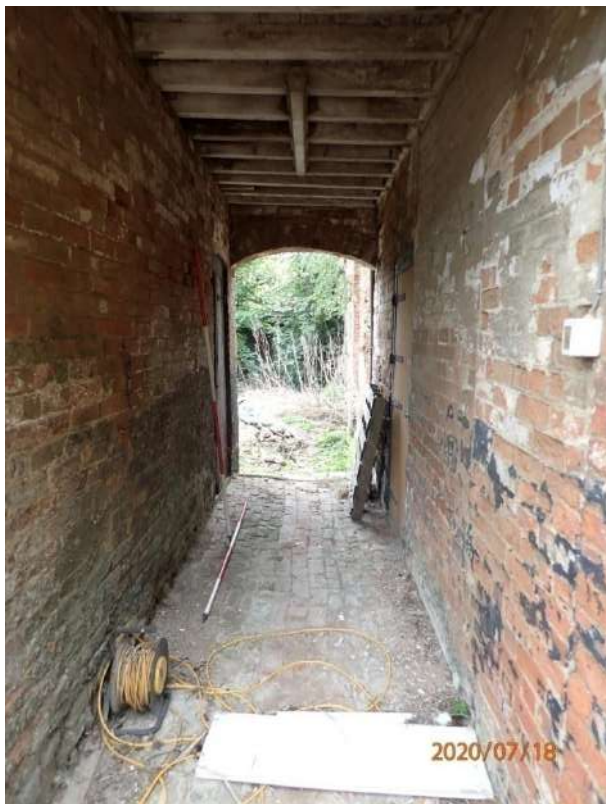
Plate 186: General view of the interior of the northern tunnel within the East Range, from the east
