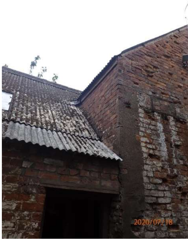
Plate 167: View of the West Elevation of the East Range, from the south
