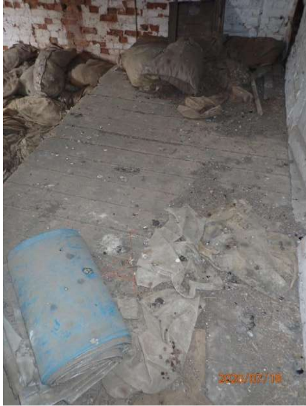
Plate 374: View of the timber platform at the northern end of Cell 17, from the east
