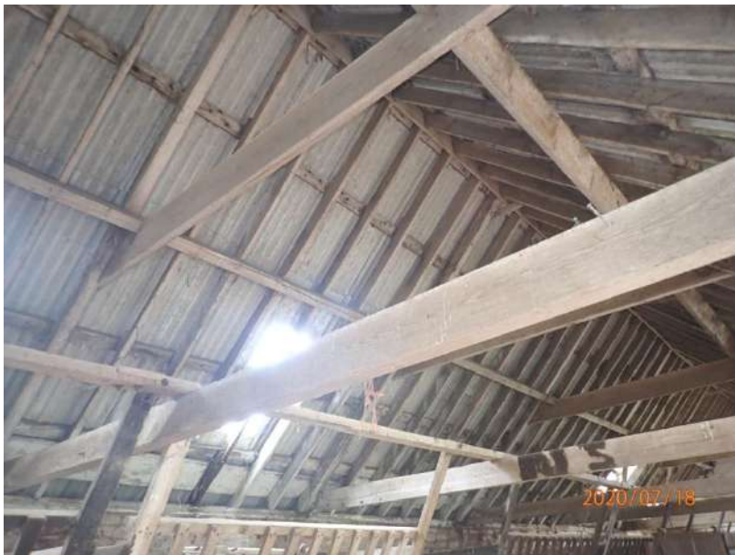
Plate 437: View of the roof supporting structure of the South Range, from the east
