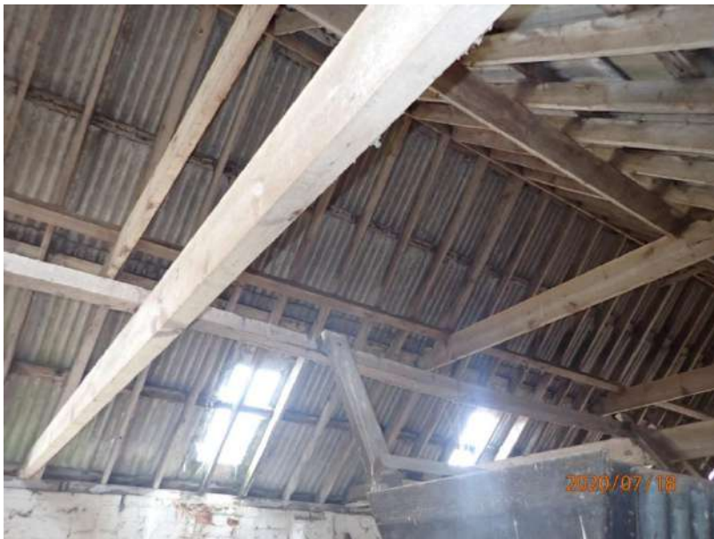
Plate 429: View of the roof supporting structure of the South Range, from the south
