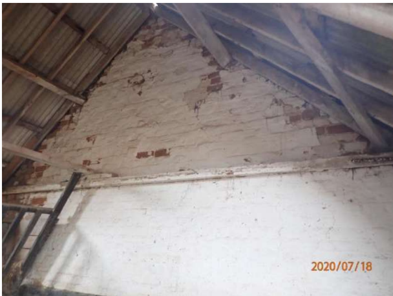
Plate 419: View of the west wall of the South Range, from the east
