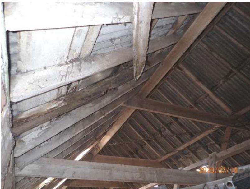
Plate 431: View of the roof supporting structure of the South Range, from the east
