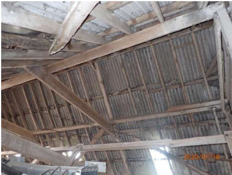
Plate 432: View of the roof supporting structure of the South Range, from the south
