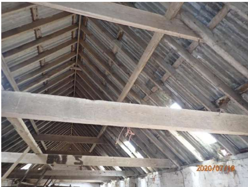
Plate 435: View of the roof supporting structure of the South Range, from the west
