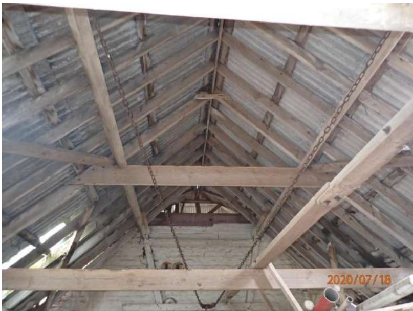
Plate 439: View of the roof supporting structure of the South Range, from the west
