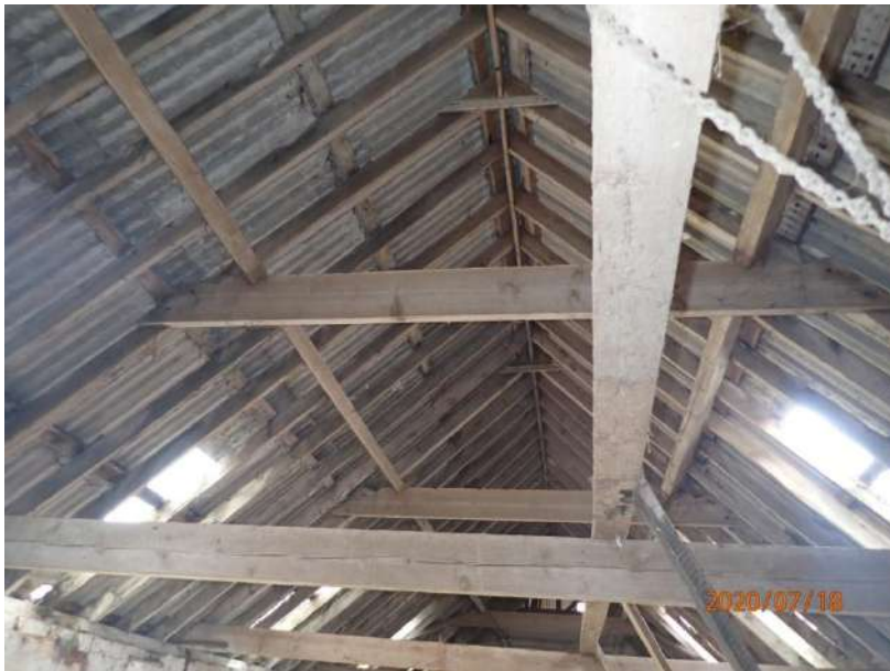
Plate 434: View of the roof supporting structure of the South Range, from the west
