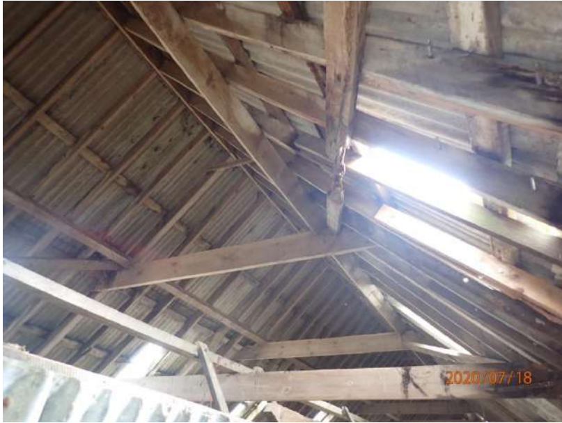
Plate 424: View of the roof supporting structure of the South Range, from the west
