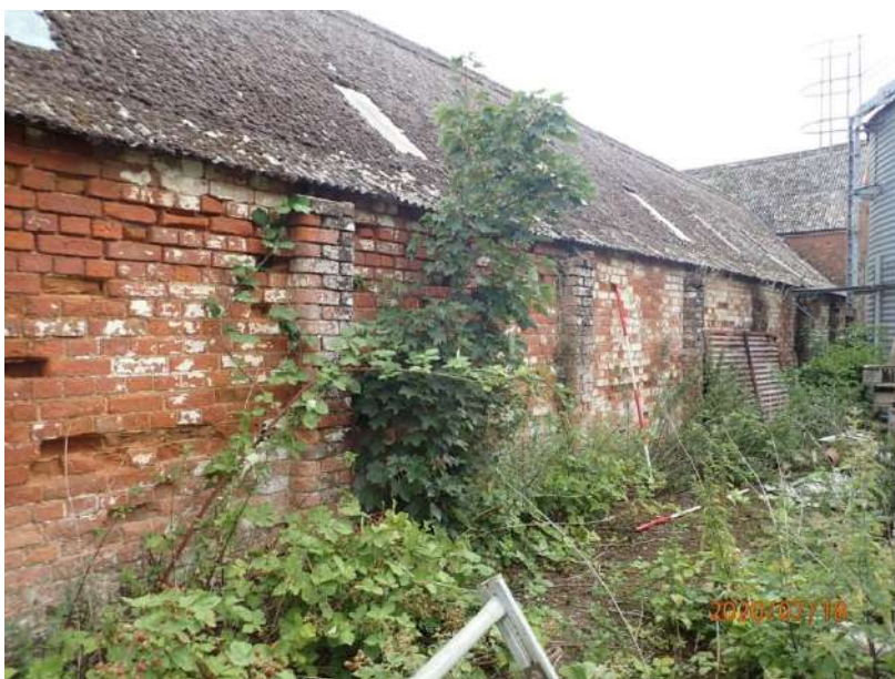
Plate 387: View of the South Elevation of the South Range, from the south-west
