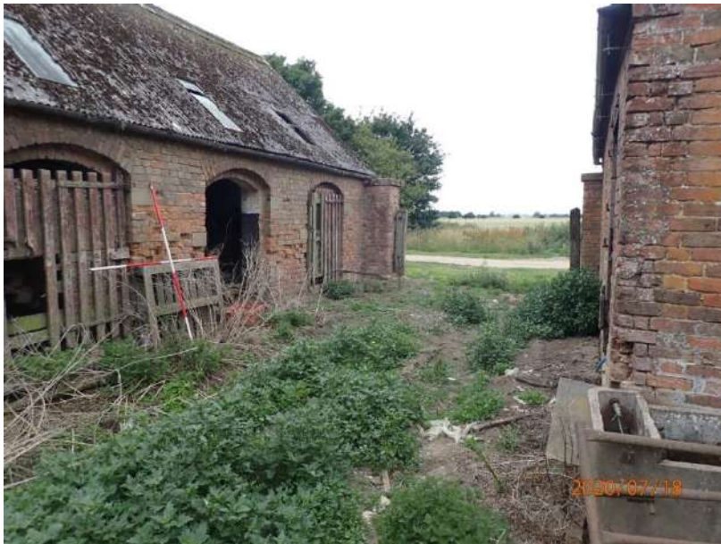
Plate 399: View of the North Elevation of the South Range, from the north-east
