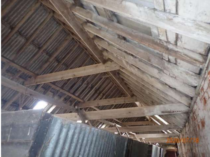
Plate 428: View of the roof supporting structure of the South Range, from the west
