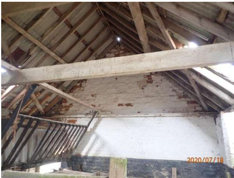
Plate 417: View of the west wall of the South Range, from the east
