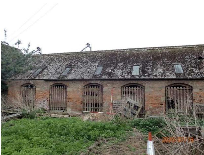
Plate 394: View of the North Elevation of the South Range, from the north
