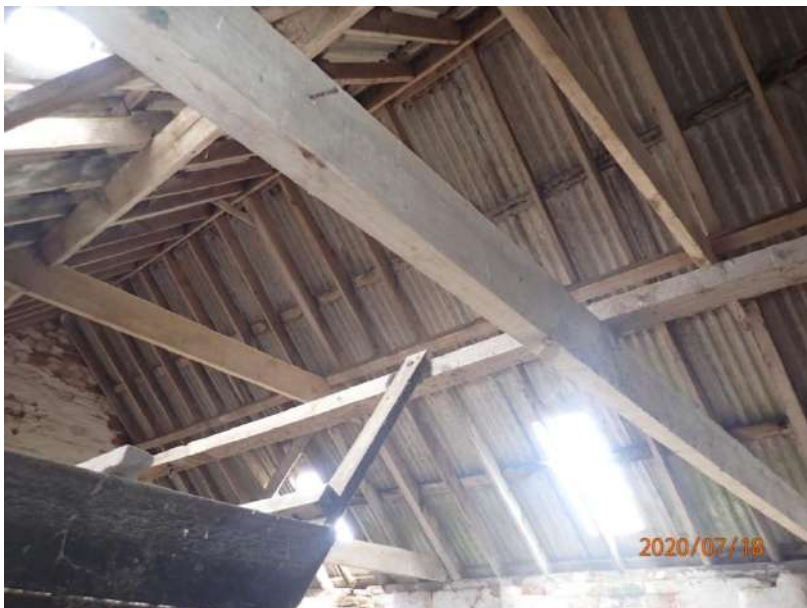
Plate 427: View of the roof supporting structure of the South Range, from the east
