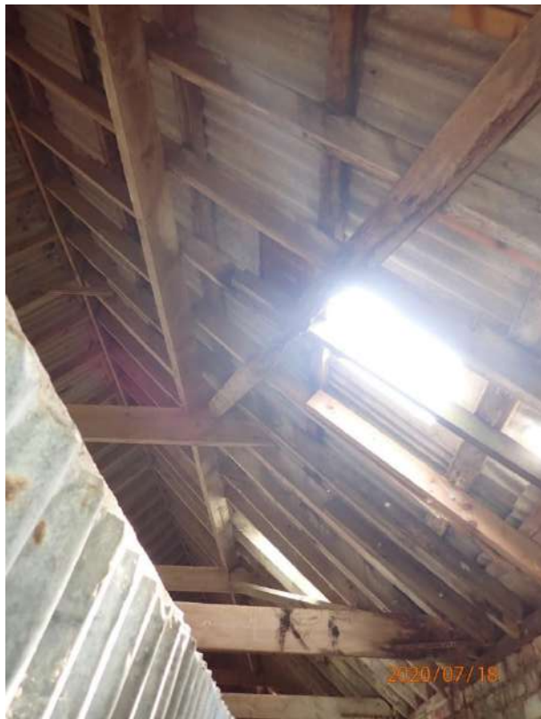
Plate 425: View of the roof supporting structure of the South Range, from the south
