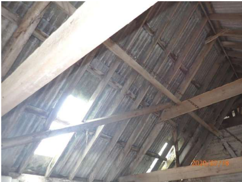
Plate 440: View of the roof supporting structure of the South Range, from the west
