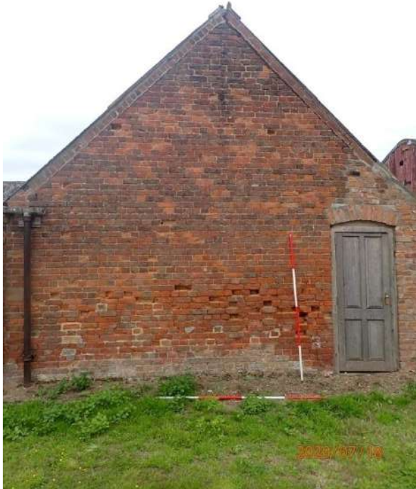
Plate 383: View of the West Elevation of the South Range, from the west
