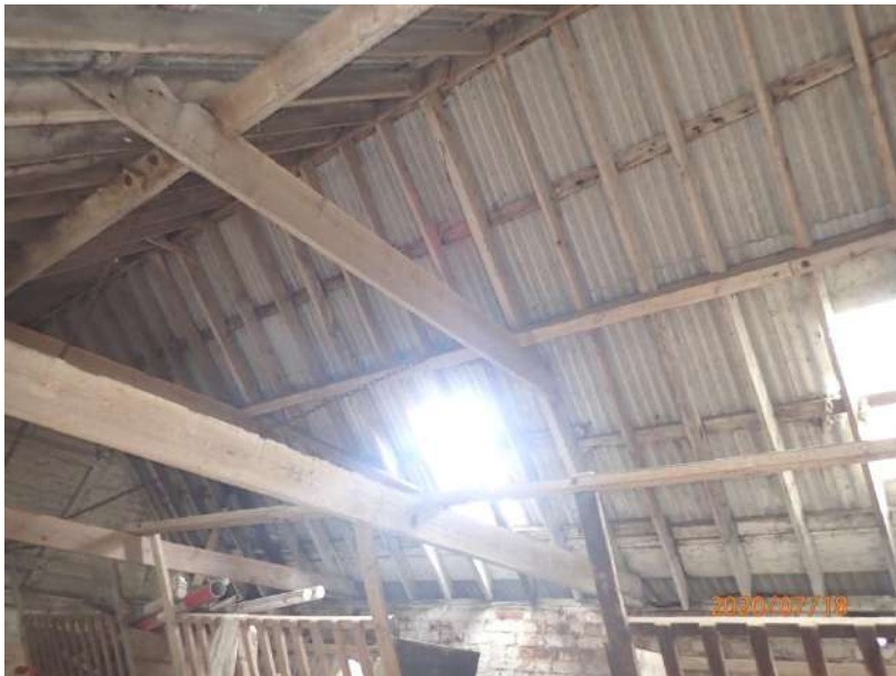
Plate 438: View of the roof supporting structure of the South Range, from the west
