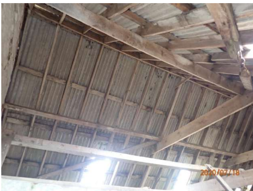
Plate 423: View of the roof supporting structure of the South Range, from the south-west
