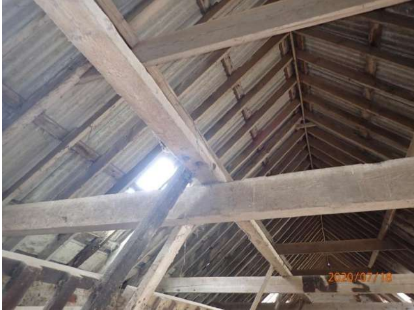
Plate 436: View of the roof supporting structure of the South Range, from the east
