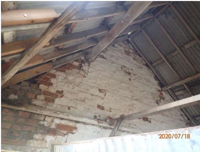
Plate 416: View of the west wall of the South Range, from the east
