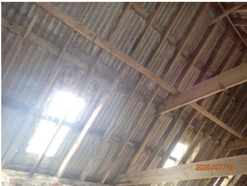
Plate 433: View of the roof supporting structure of the South Range, from the west
