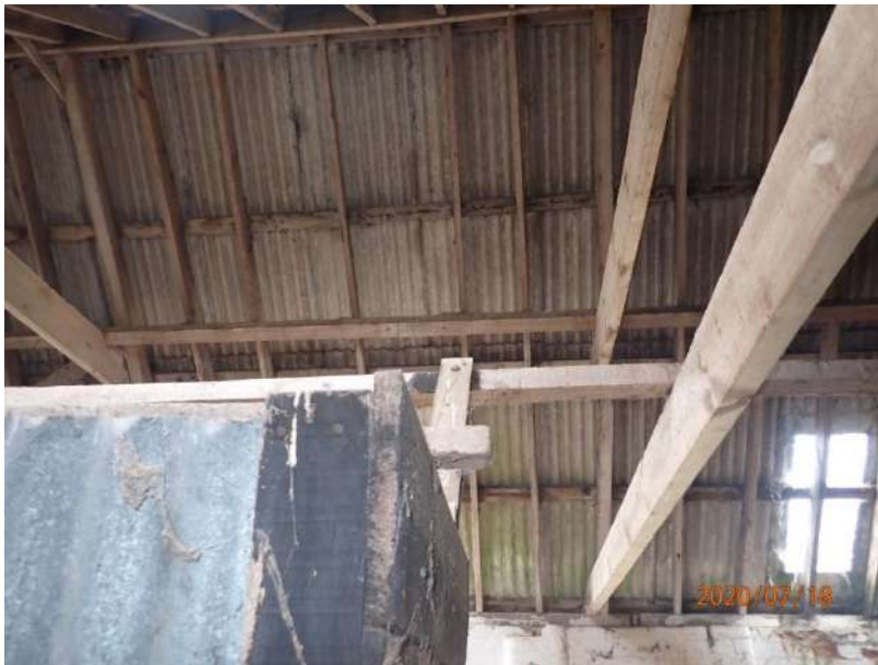
Plate 430: View of the roof supporting structure of the South Range, from the south
