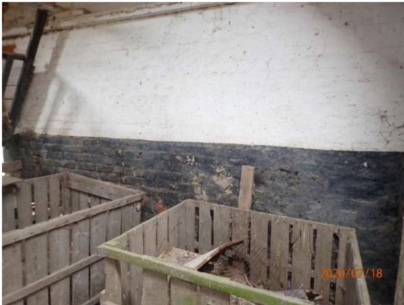
Plate 418: View of the west wall of the South Range, from the east
