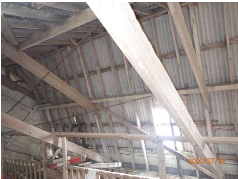
Plate 441: View of the roof supporting structure of the South Range, from the west
