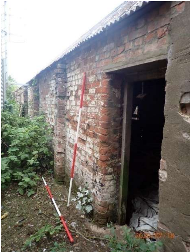
Plate 392: View of the South Elevation of the South Range, from the east
