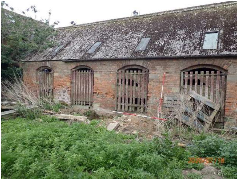
Plate 395: View of the North Elevation of the South Range, from the north
