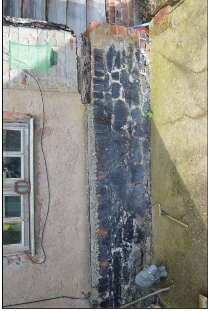
Fig. 26: Stone and brick plinth at the north-east corner of the house (CPAT 4900-0020)
