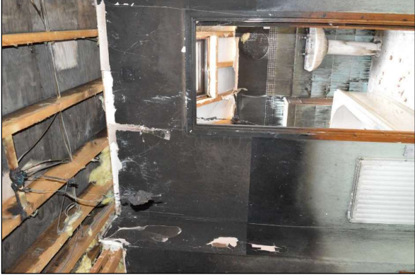
Fig. 50: Fire damaged landing and bathroom (CPAT 4900-0044)
