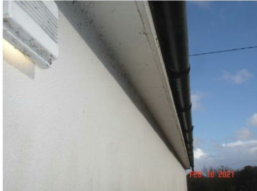
Photograph 2 – View of the soffits on the garage building.
