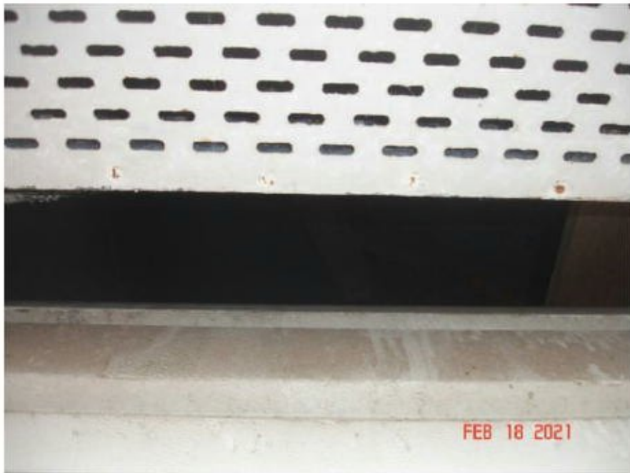
Photograph 3 – View of the large gap at the top of the metal garage door, partially blocked with material internally.
