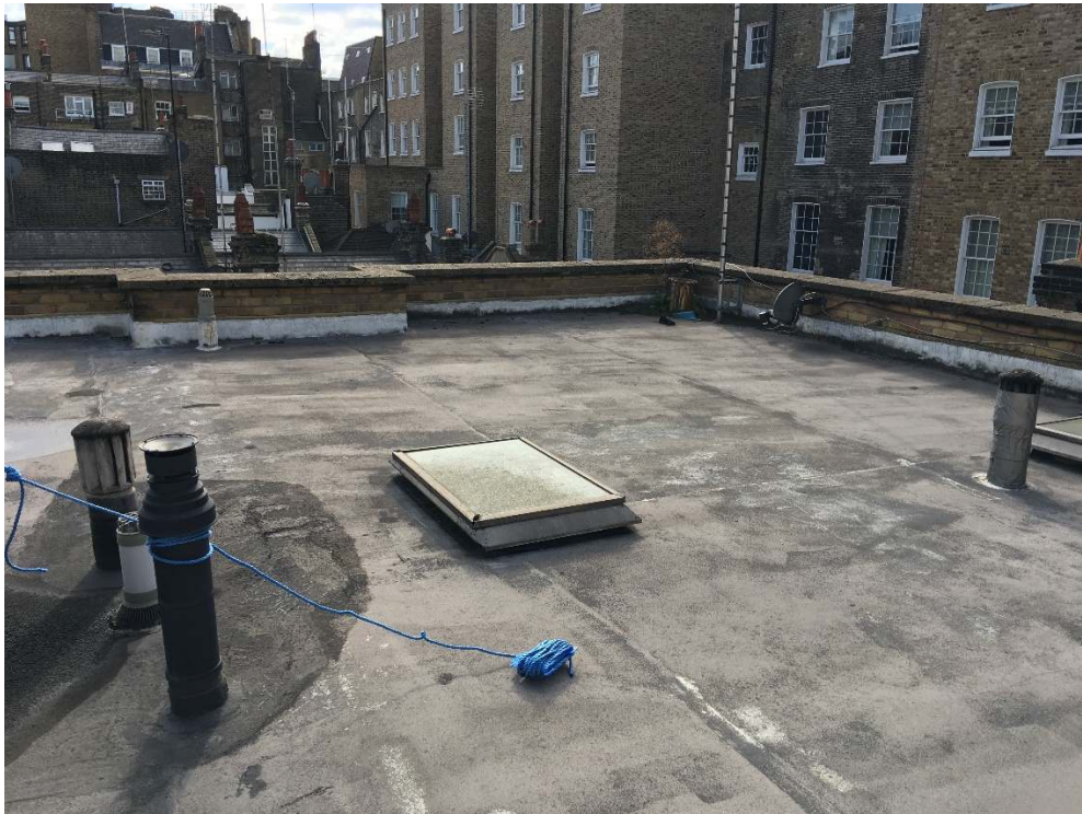
4 View South Across 3 Montagu Mews South and To Rear of Gt Cumberland St
