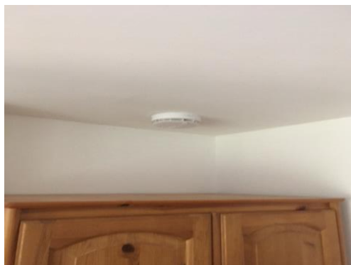
Figure 1 Smoke detector head to close to wall.
