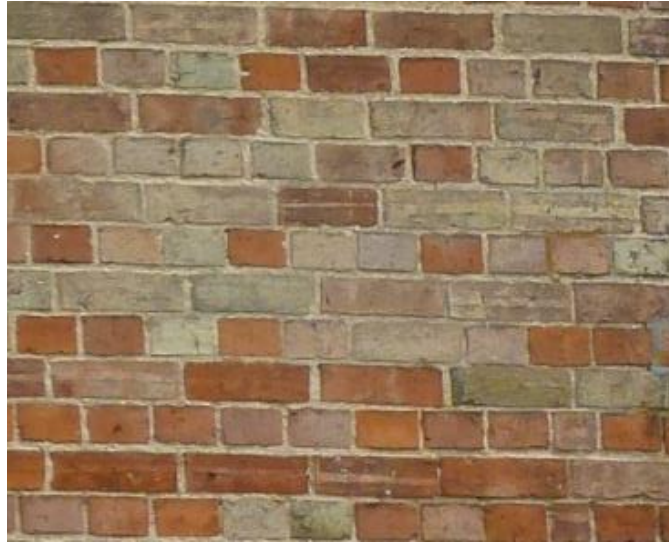
Above: traditional English bond brickwork which is typical of the buildings and structures on the site.
