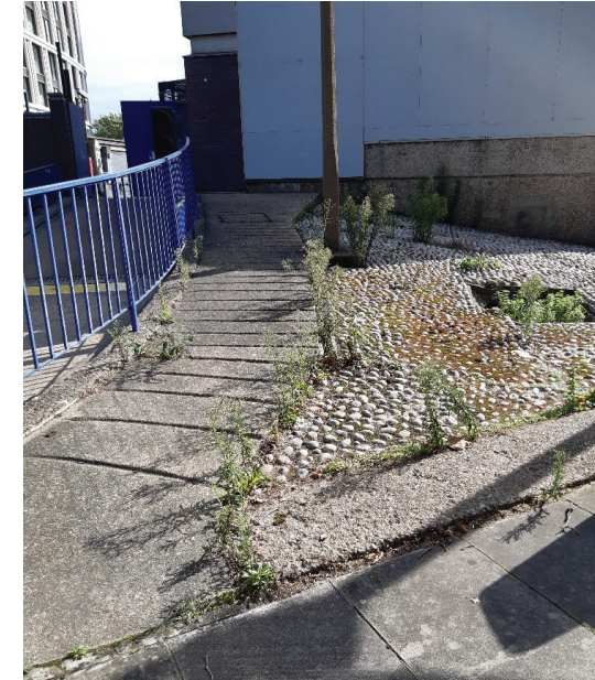
Photo 5. Example of ephemeral vegetation growing in unmanaged paving cracks, in west of site.
