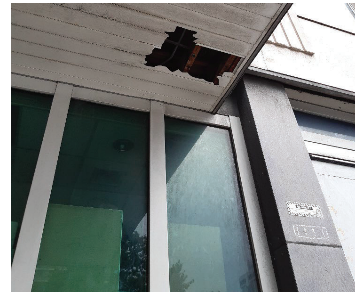
Photo 6. Example of gaps into building, with damaged underside of porch at main entrance on south-east corner of site. Not considered to be suitable for roosting due to site setting.
