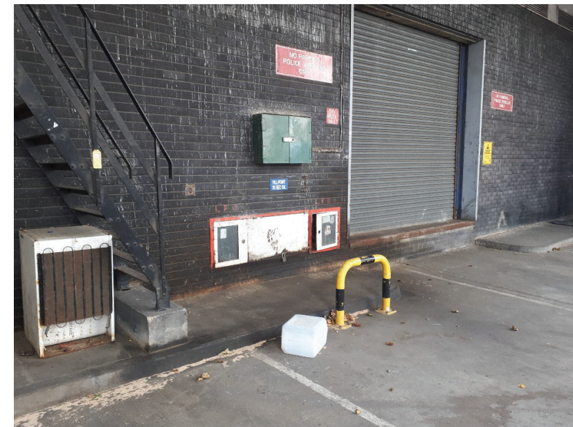
Photo 6. Tank fill point in the east of the site, likely associated with oil fuel heaters formerly located in the eastern extent of the basement.
