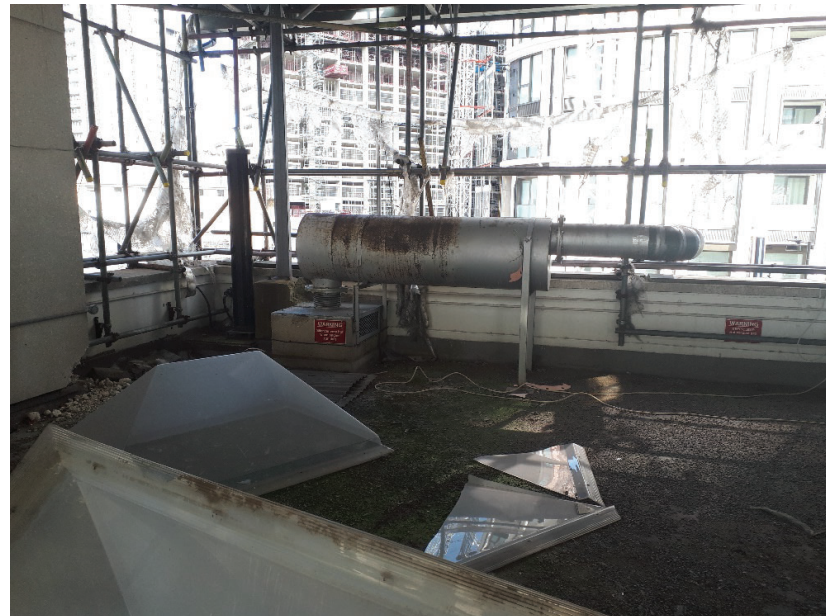
Photo 8. A 'silencer' and associated generator on the flat roof of the elongated low-rise structure connecting the eastern and western towers.
