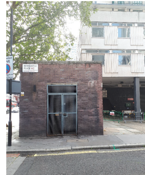
Photo 10. Electricity substation in the north-eastern corner of the site on Newcastle Place.
