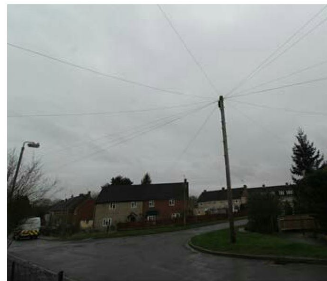
[Figure 40] Overhead cables and post
