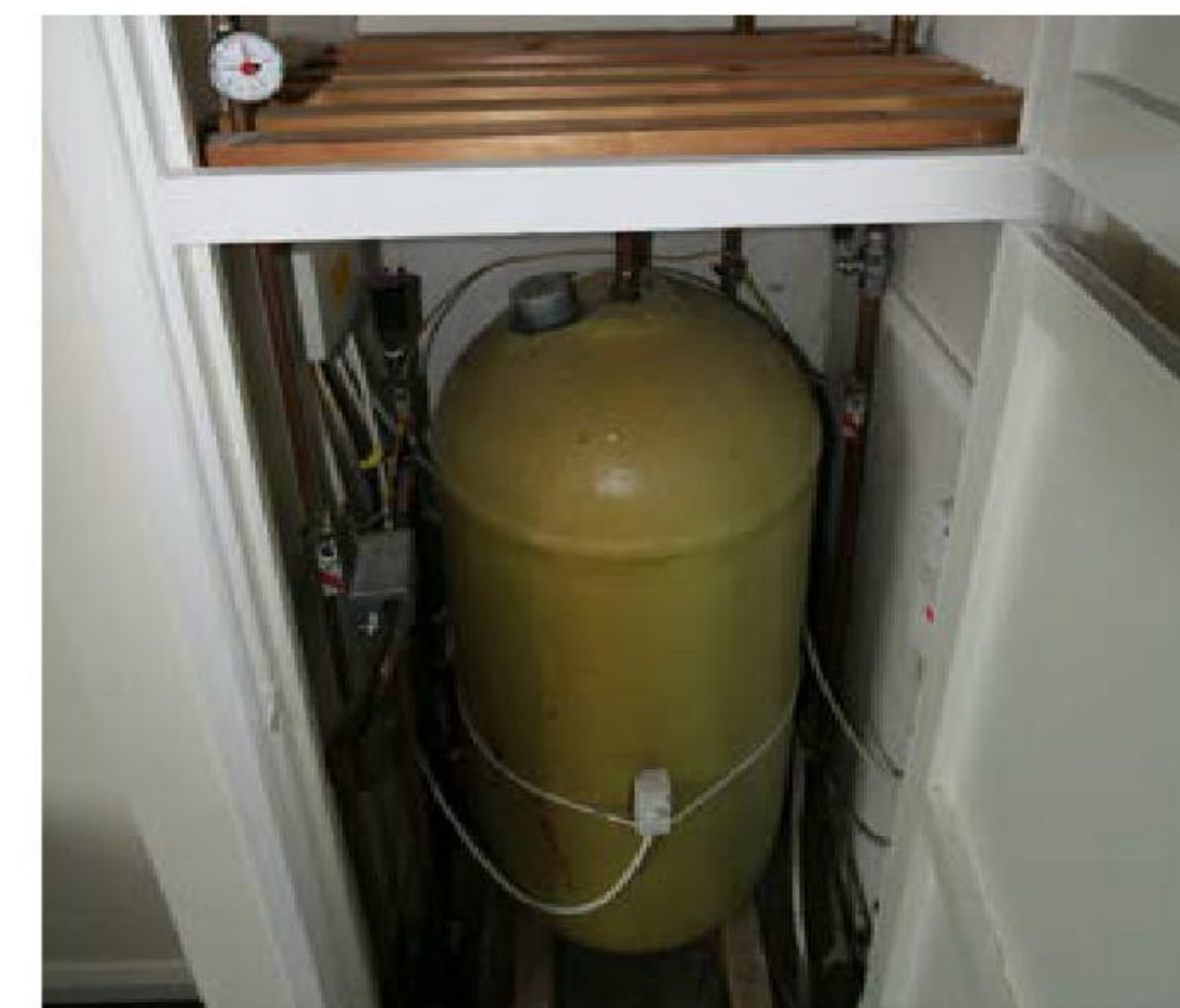
[Figure 34] Hot water tank in bedroom 1
