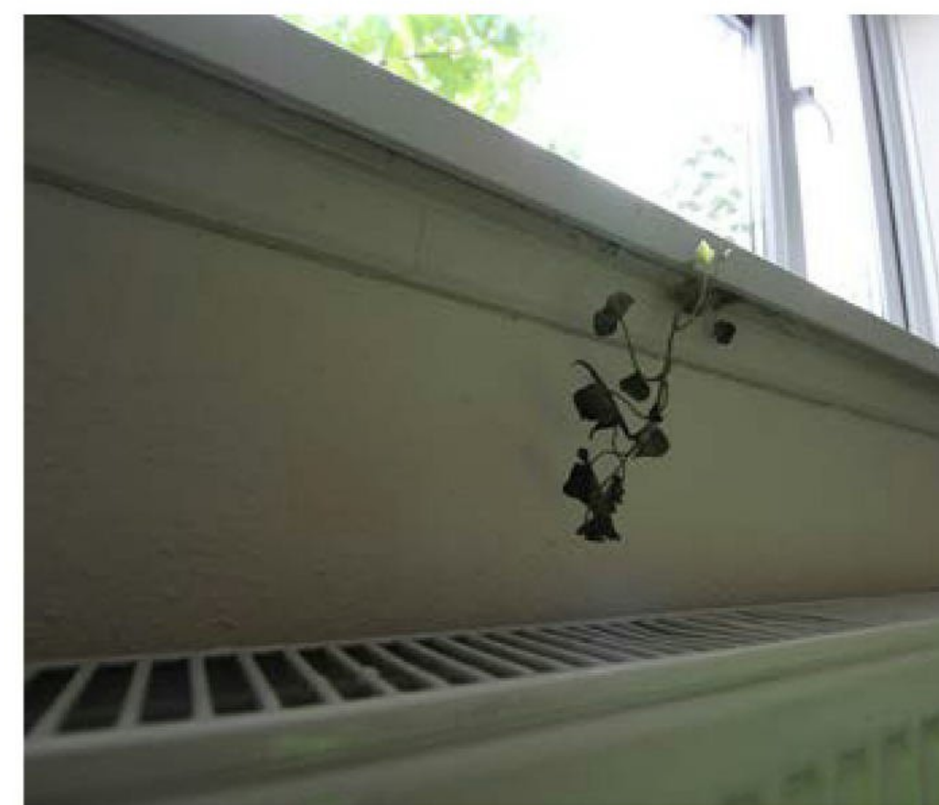
[Figure 44] Ivy ingress through living room
