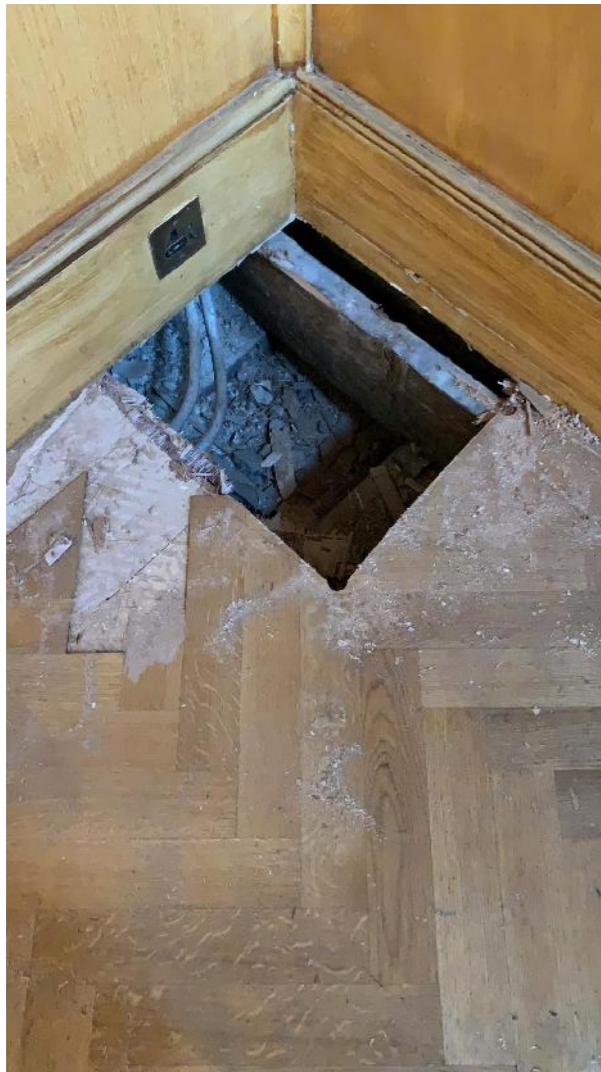
1 layer of Timber harring bone 1 layer of ply Joists 240X50 Some damages to joists
