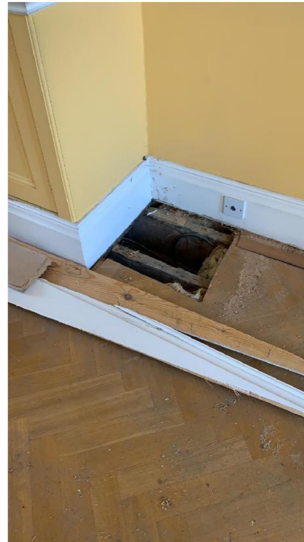
1 layer of Timber harring bone 1 layer of ply Joists 140X70 Some damages to joists
