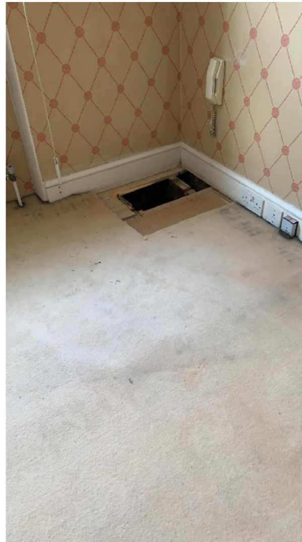
1 layer of Carpet 1 layer of pine boards of recent manufacture Joists 200X60 Some damages to joists
