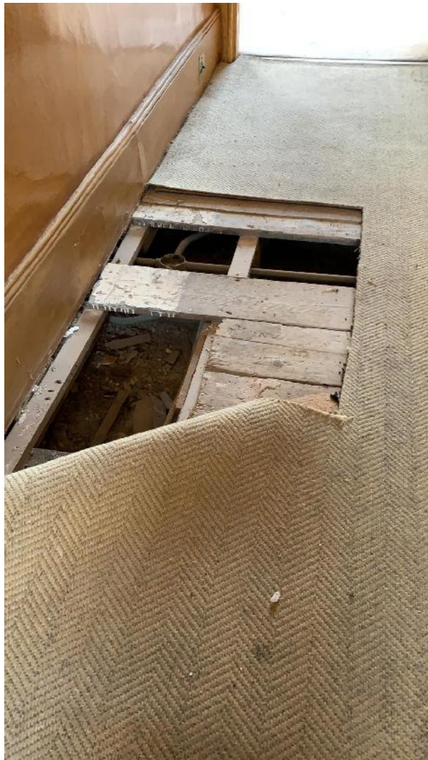
1 layer of Carpet 1 layer of ply pine boards of recent manufacture Firrings Joists 200X60 Some damages to joists
