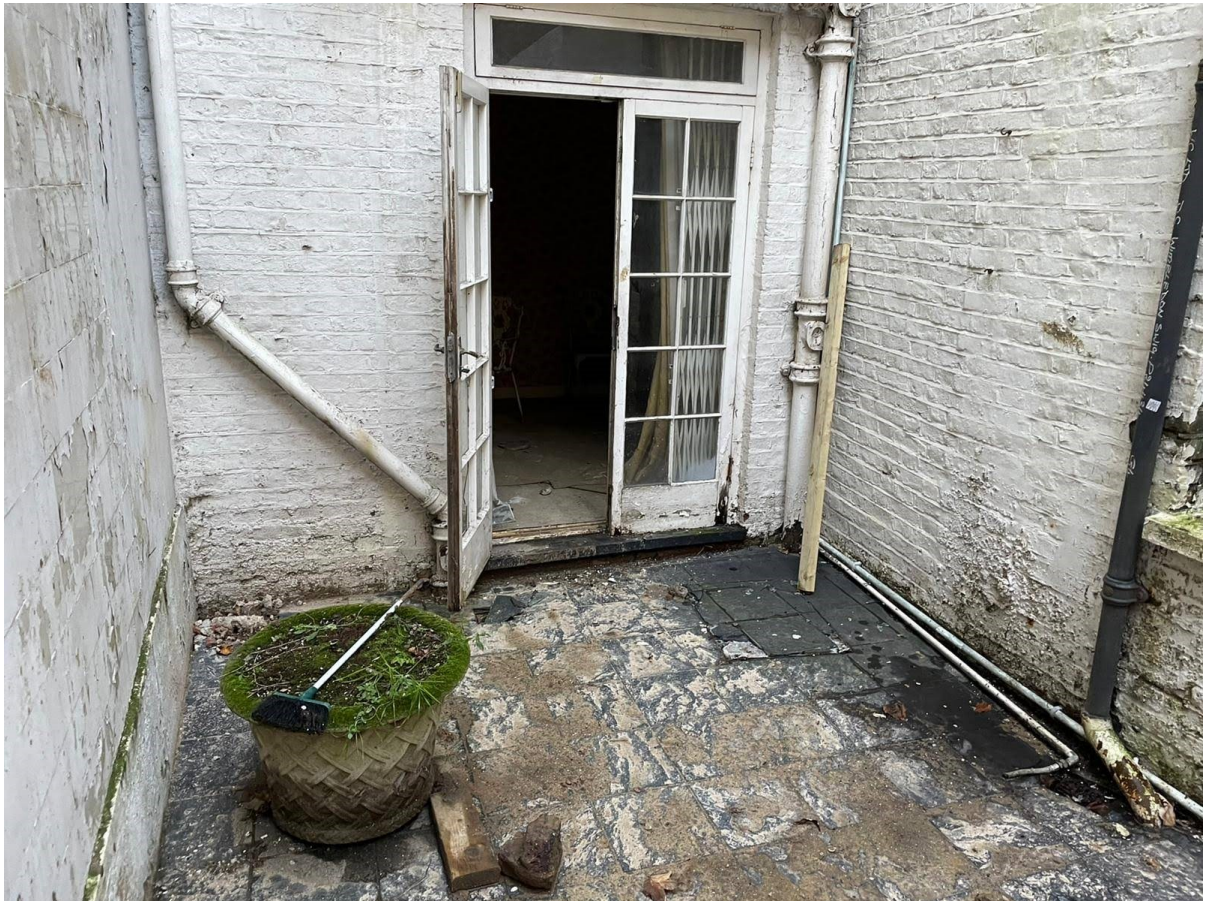
Photograph 9: Basement level at the rear of the building, facing towards the east.
