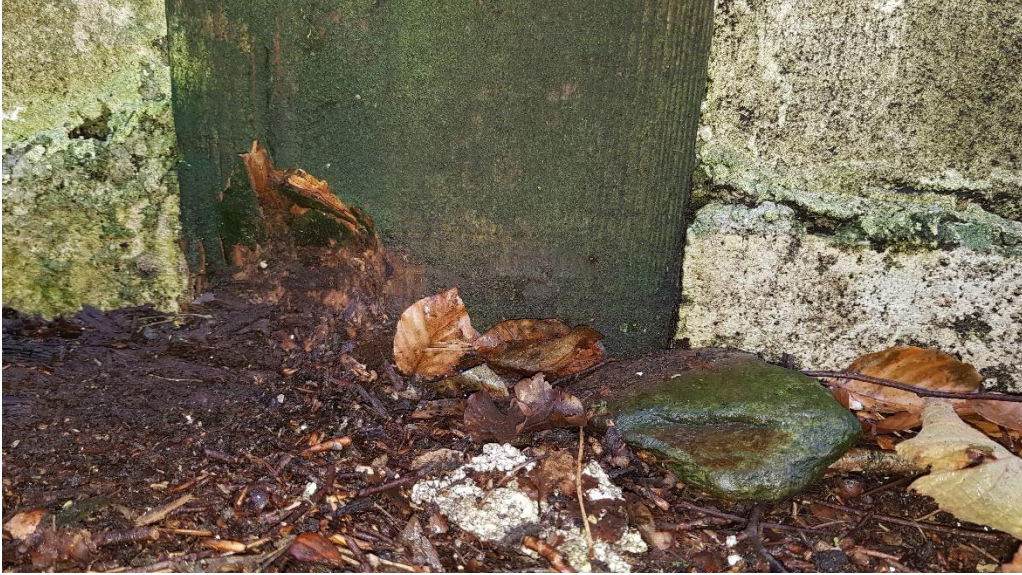
Photograph 3. Rotten timber at bottom of post
