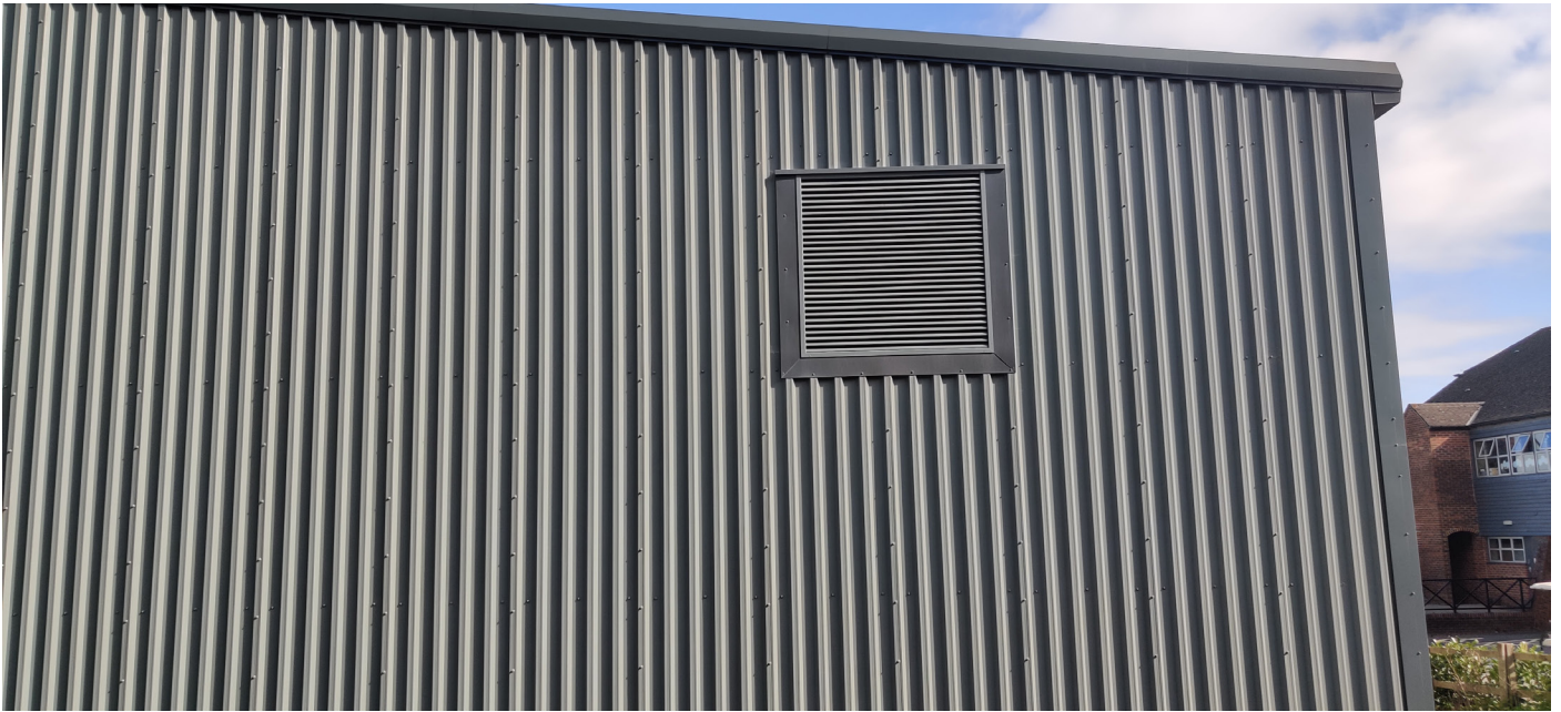
Photograph No. 1 - View of the existing sports hall (B1) which is to be extended within the proposed development.
