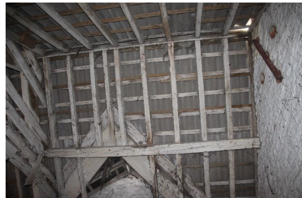
6. Unlined roof of NE building at join with stock shed
