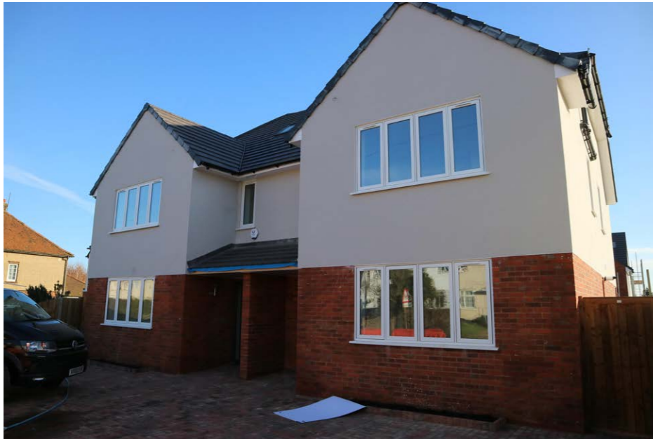
New Development Under Construction - 50-53 Chesham Road Materials - Brick and Render Elevations with White Fenestration and a Grey Roof Tile
