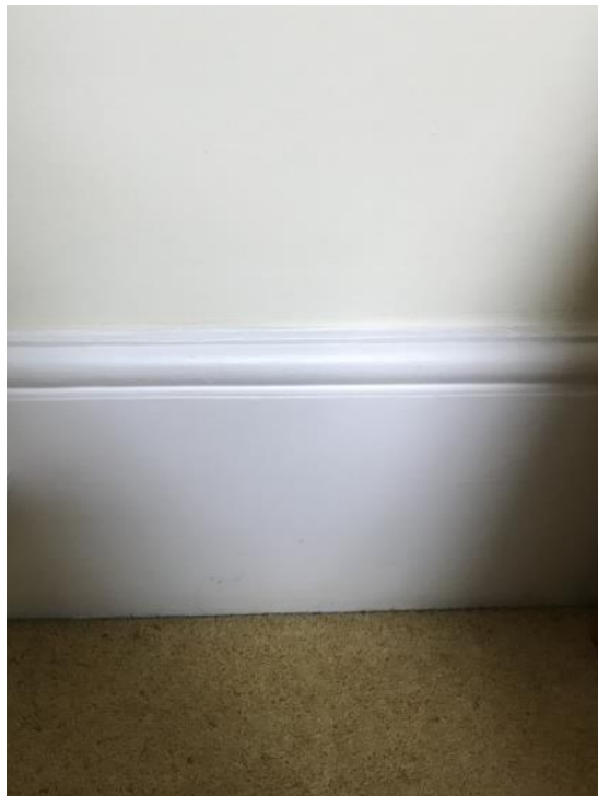
SKIRTING THROUGHOUT—LIKELY NOT ORIGINAL
