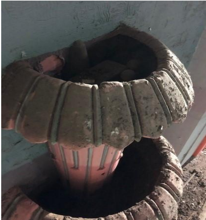
Fountain cover in dirt.
