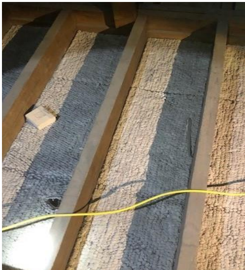
Rear of Main Flat Bed Ceiling – Sound Plaster Key.
