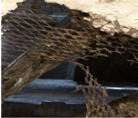
Rotten timber & corroded metal lath.
