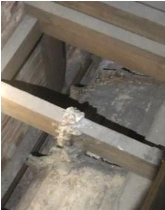
Wads inspected on the mouldings running across the front the Proscenium check & in good condition.
