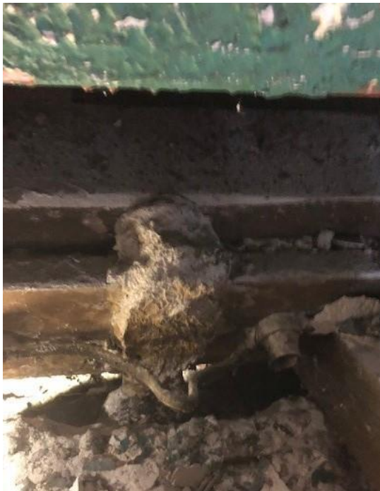
Bea & Reel light trough – Wads rotting
