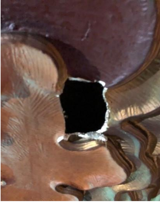
Damage to Freize.
