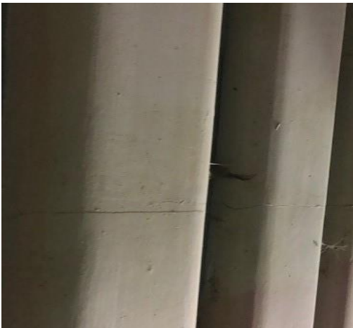
Panel 3 – Crack along casting joint
