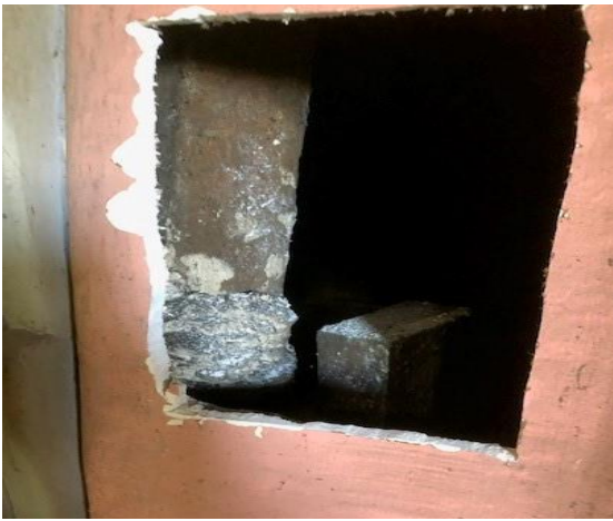
Rotten wad viewed through inspection hole.
