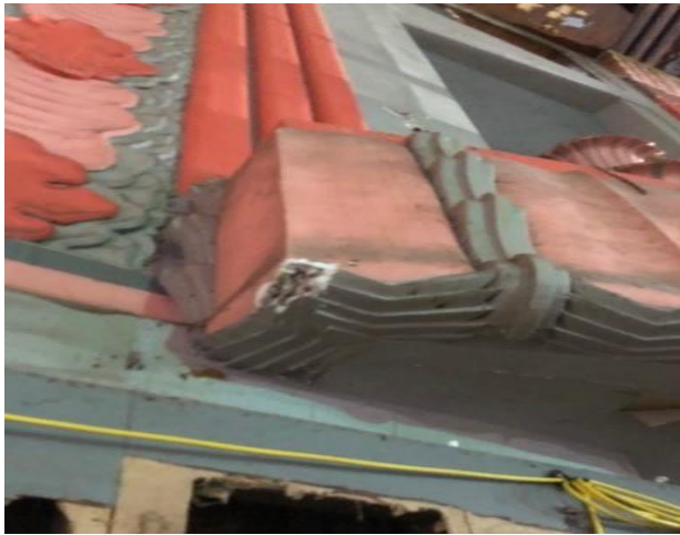
Chipped corner to base moulding
