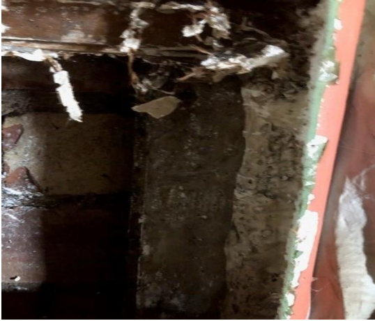
Decayed hessian in back of cast caused by water ingress.
