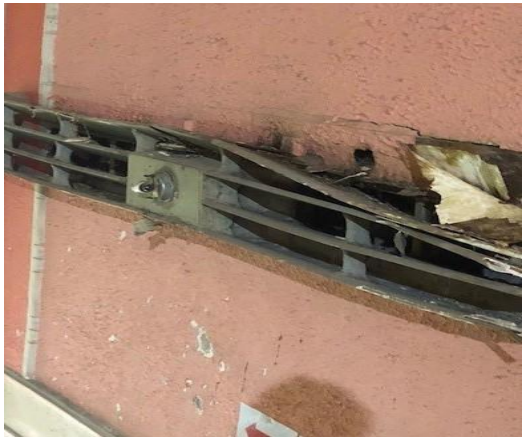
Grille damaged beyond repair
