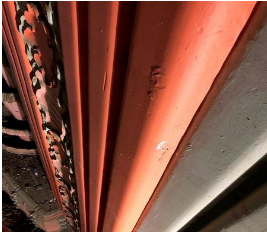
Minor damage to ribs.
