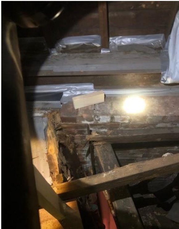
Rotting timber joists.
