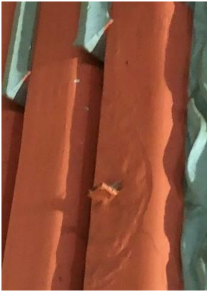
Metal intrusions in panel. 4nr each side of auditorium
