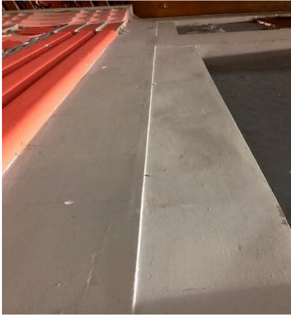
Panel with minor damage
