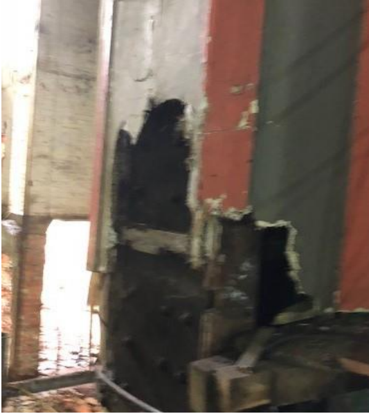
Damage to base of Arch Stage Left
