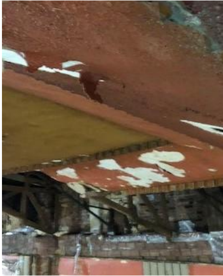
Missing Sloping Sections
