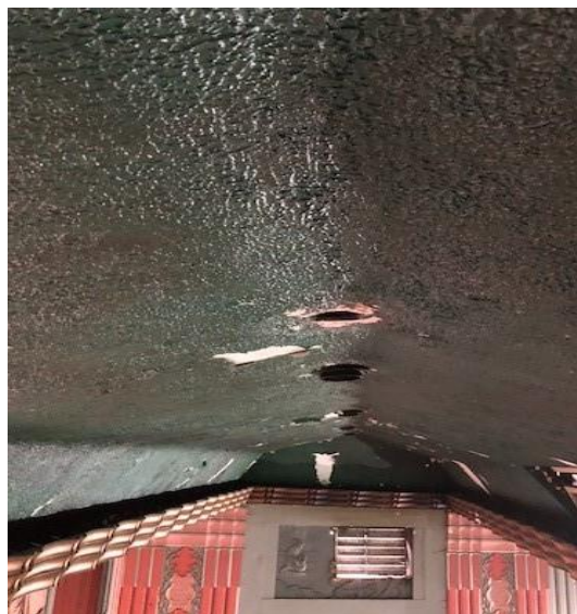
Face of vaulted ceiling – Minor localized repairs
