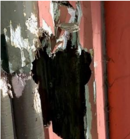
Damage to sides of Proscenium Arch stage left.
