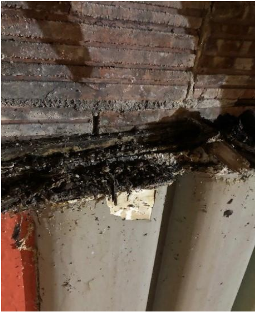
Panel 2, water has got into the back of the ribs & caused the hessian & timber to rot.
