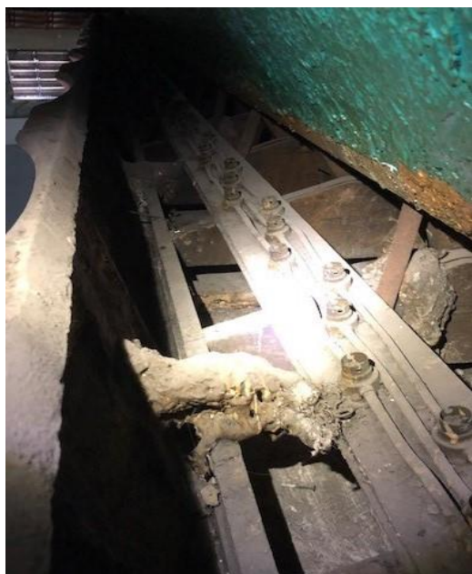
“Wad” rotting in lighting trough
