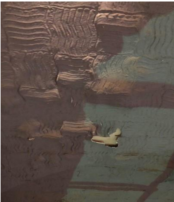
Background wall Fountain fixed to. Textured coating de-bonding.
