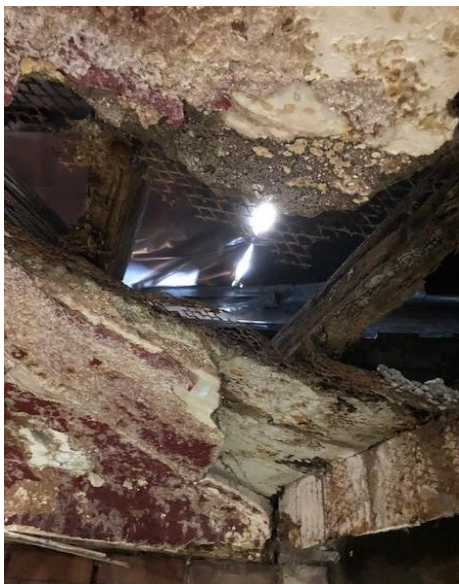
Close up section of badly damaged sloping ceiling. Rotten timber & corrosion to metal lath. Stage right GL4
