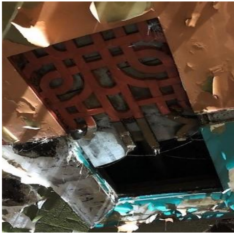
Damaged grille. Can be reproduced off site & replaced.
