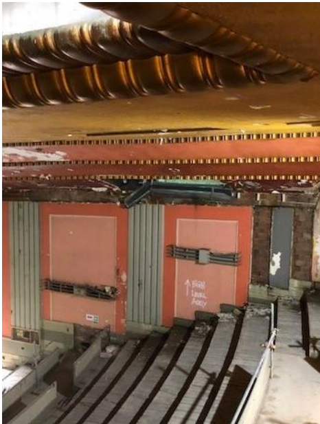
Panel 1 – missing, Panel 2 – rotten, Panel 3 – Minor damage.
