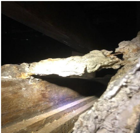
Wad holding cornice rotten & wire corroded.
