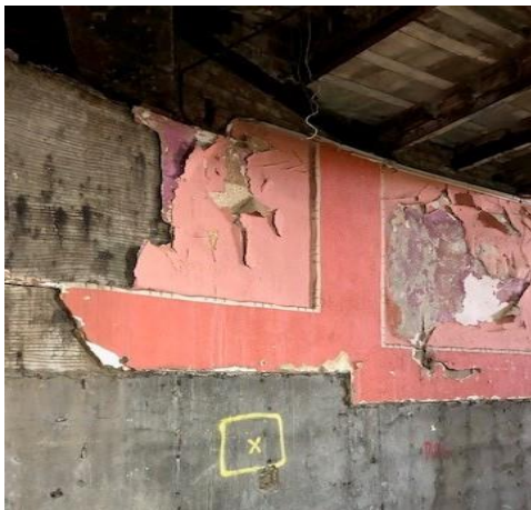
The traditional , Lime putty plaster to the walls is missing in all locations except the small amount shown. This loose & crumbling. It should be removed. It can however, be replaced to match existing with the panel mouldings reproduced off site.
