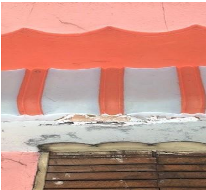
Vertical down stand Moulding – 230mm. Fixed on cantilever timber frame work. Manufactured off site. Slight damage to one section , repairable on site. General good condition in other places.
