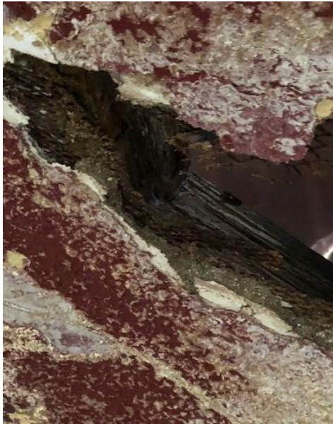
Rotten & corroded section, stage left GL 7-8
