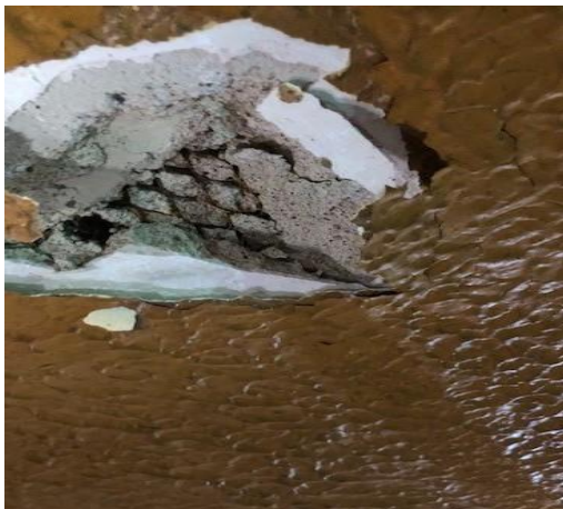
Face of Main flat bed ceiling – Localised damage.
