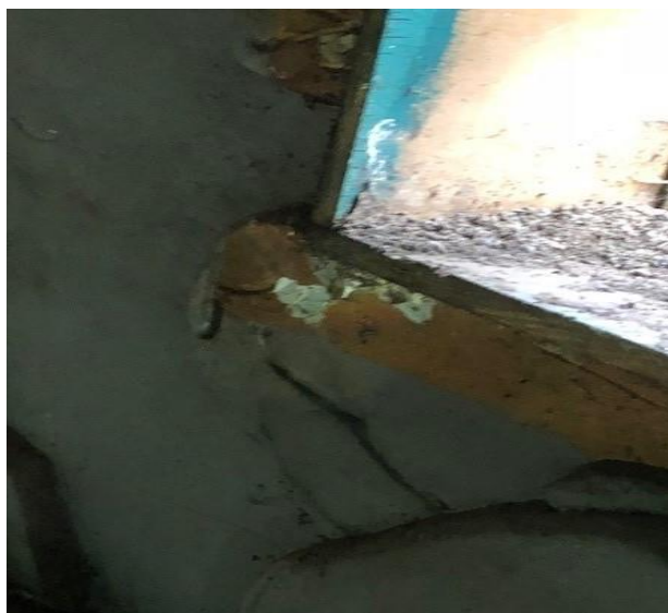
Damage to Entablature Panel
