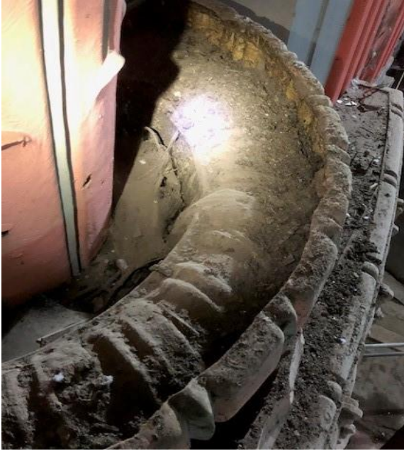
View inside of the Fountain, chipped edges, dirt.
