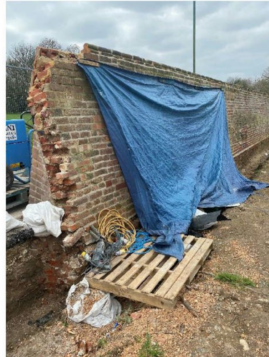
Ready to be toothed out and new wall starter per the specification
