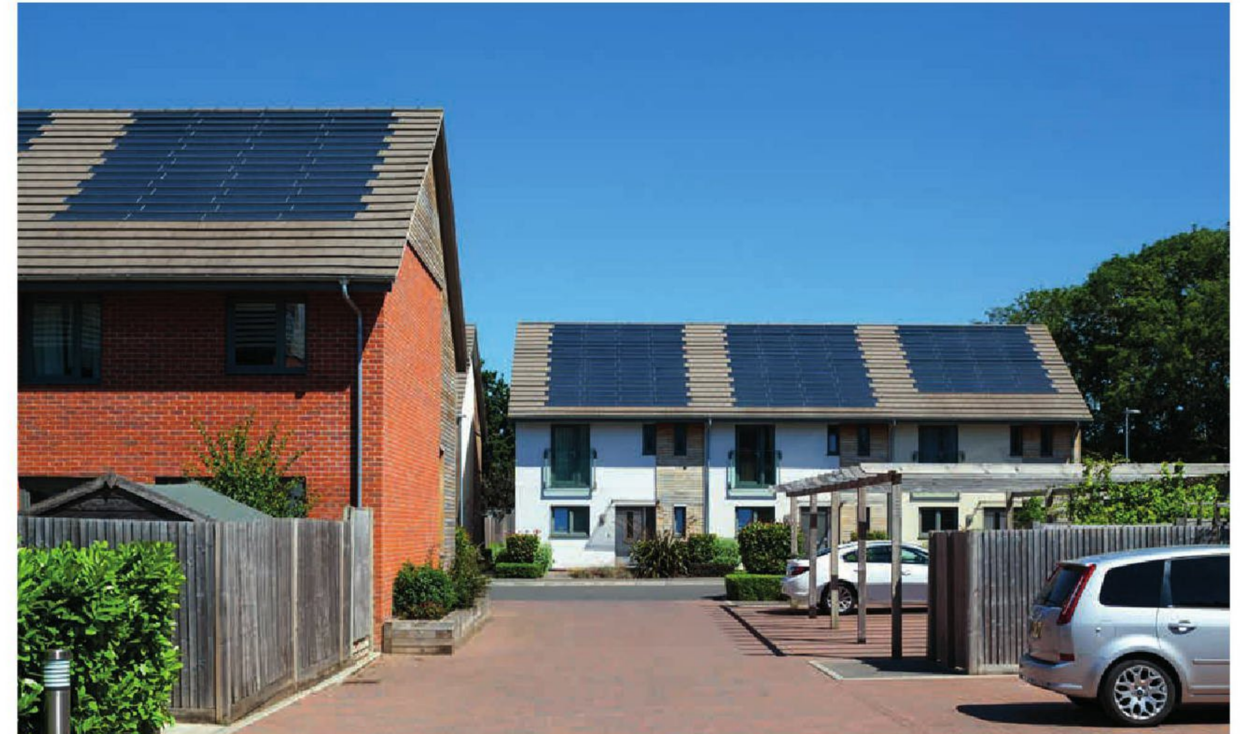
Solar PV system integrated into the roof tiles at Graylingwell, Chichester
