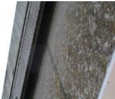
Plate 4.11: Gap behind fascia board
