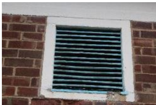
Plate 4.15: Vent with large gaps
