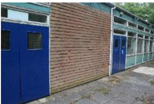
Plate 4.7: Broken, dislodged and missing hanging tiles
