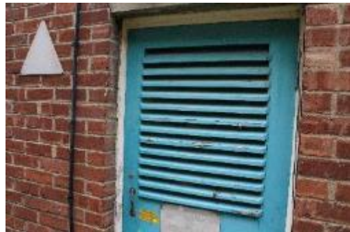
Plate 4.14: Louvre door with large gaps
