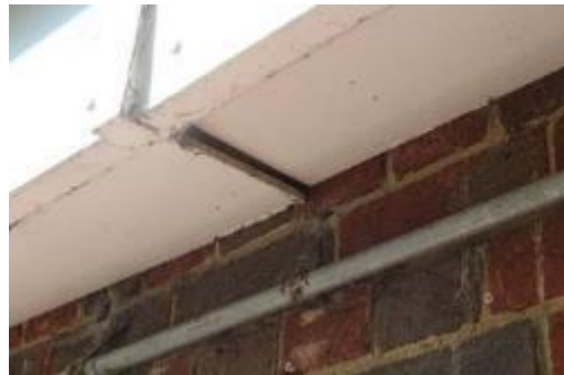
Plate 4.12: Gap in soffit
