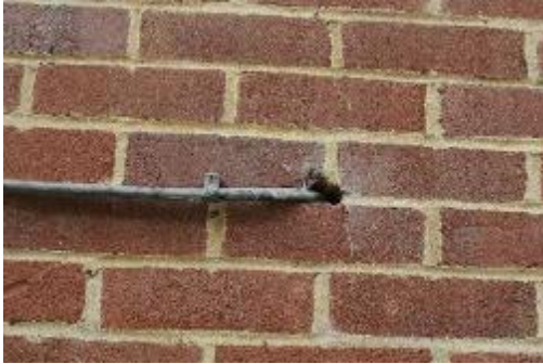
Plate 4.9: Hole in brickwork around cable inlet
