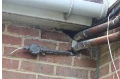
Plate 4.10: Hole in brickwork around pipework
