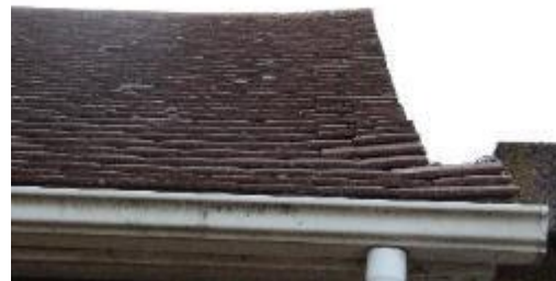
Plate 4.6: Dislodged roof tiles
