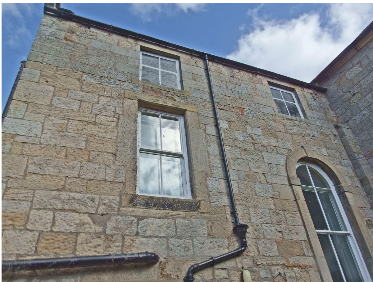
West face of the Stair Wing, showing added top floor in greyer stone
