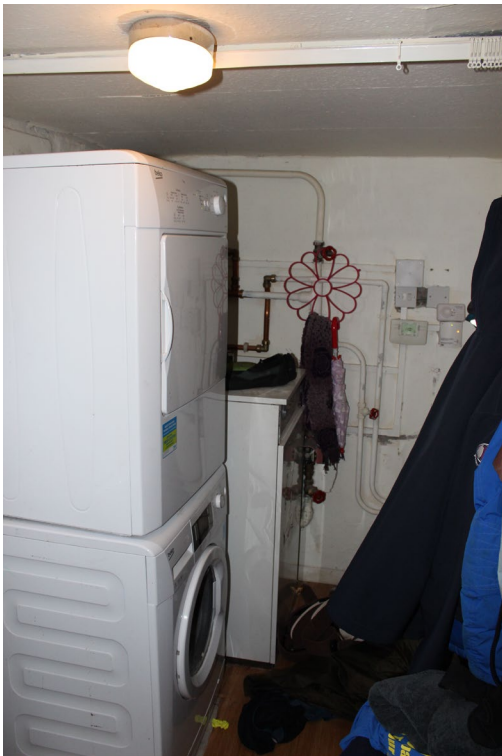
Existing wc with laundry and boiler, all to be removed and new shelving installed for the pantry.
