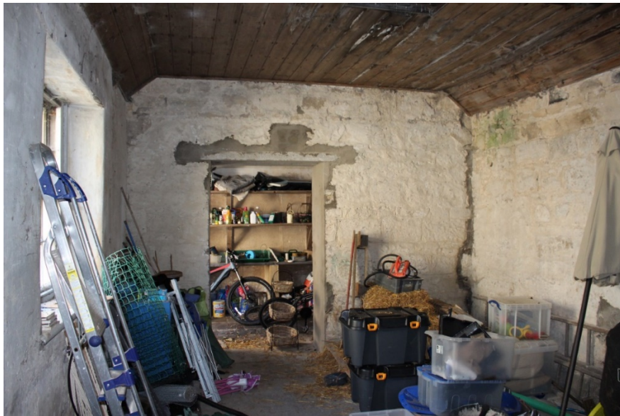
South wall of the proposed studio with existing modern opening formed in the internal wall.
