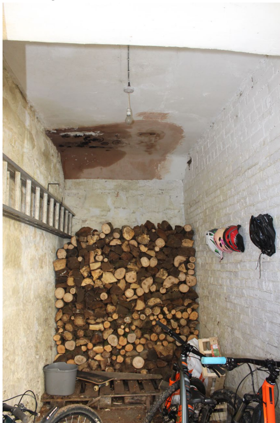
Store room to the south end with damage from water penetration.
