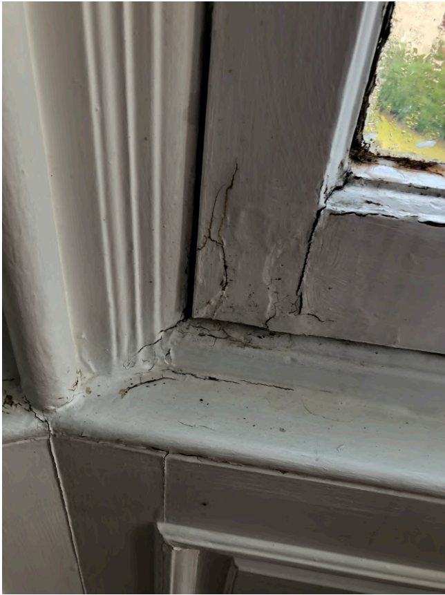
Timbers are breaking at joints
