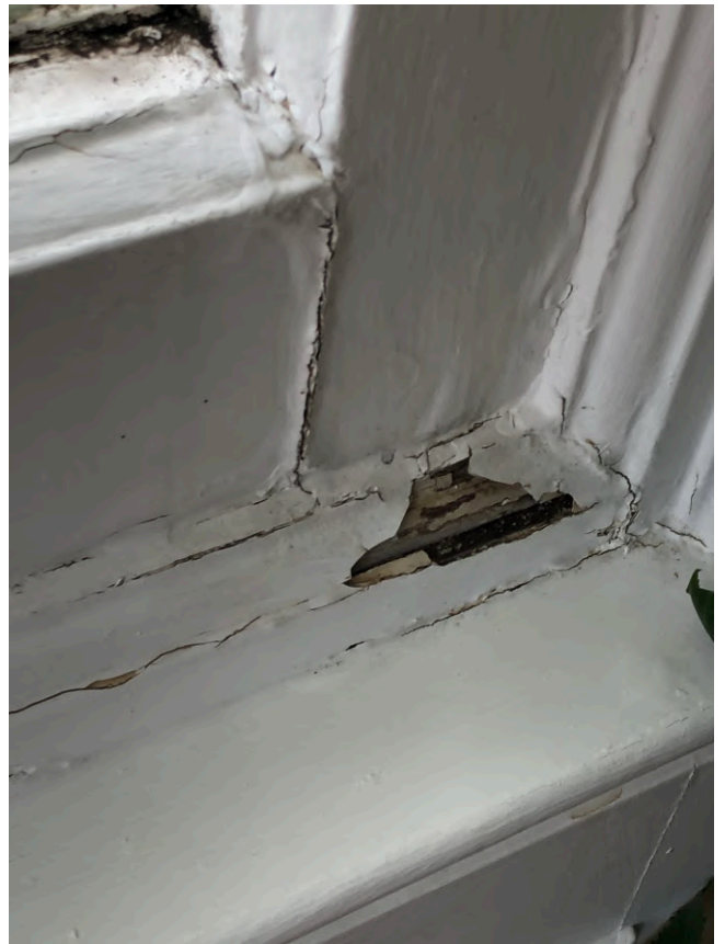
Paint work is breaking away from timbers due to rot
