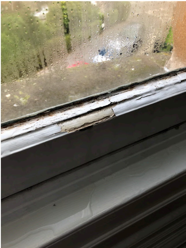
This is typically how much condensation builds, there is water sitting on the timbers which will weaken timbers even more
