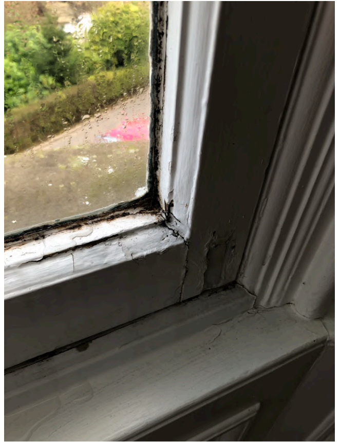
Timbers are breaking at joints
