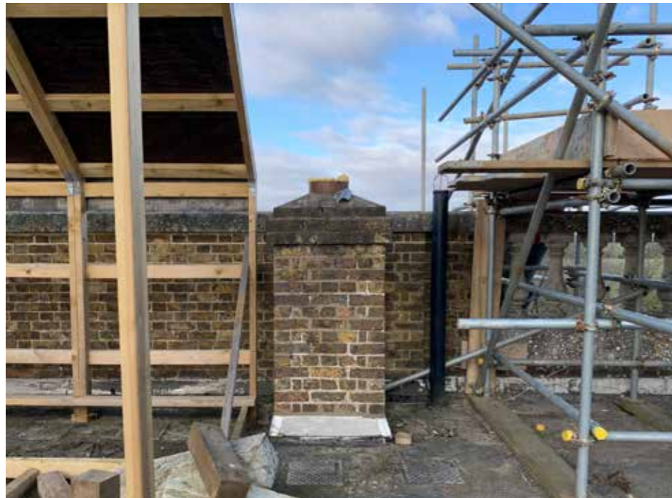
Plate : 23 Western parapet and mini chimney stack serving the Study on the Ground Floor. Consent is granted to rebuild the parapet with stone bottle balusters over the windows and incorporate this flue into the wall to comply with Building Control.
