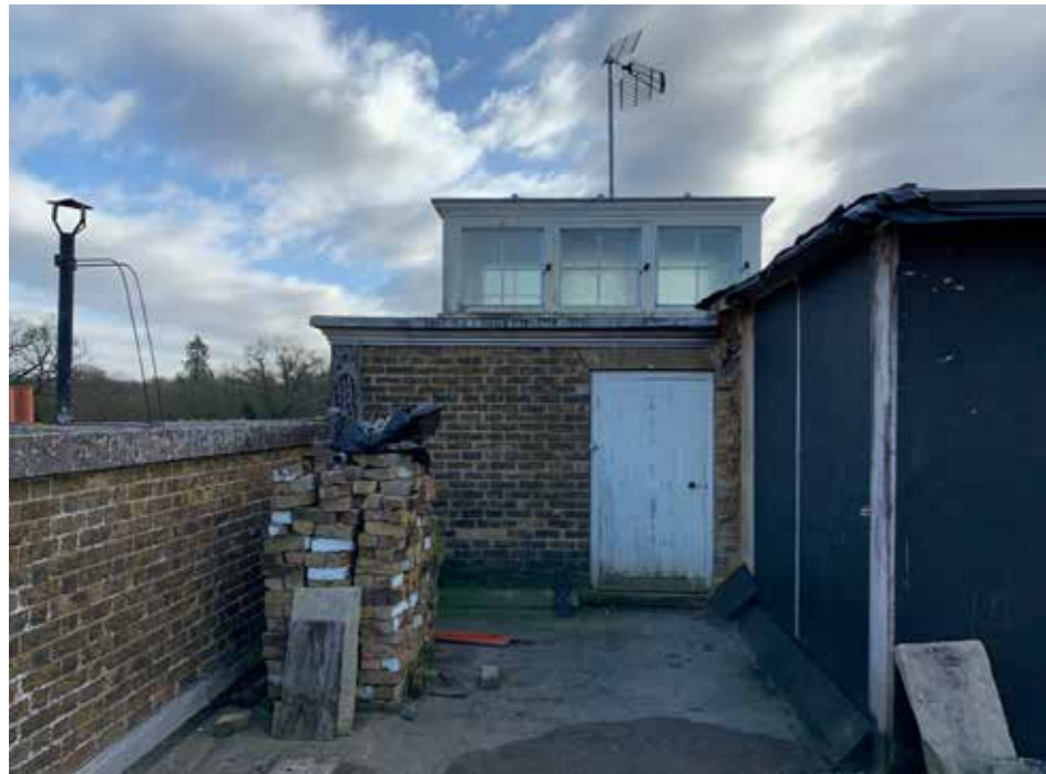
Plate : 11 Edwardian roof lantern and service door adjacent to service lift opposite north parapet. Consent is granted to remove the roof light and rebuild the parapet in a brick and pointing to match the main house.
