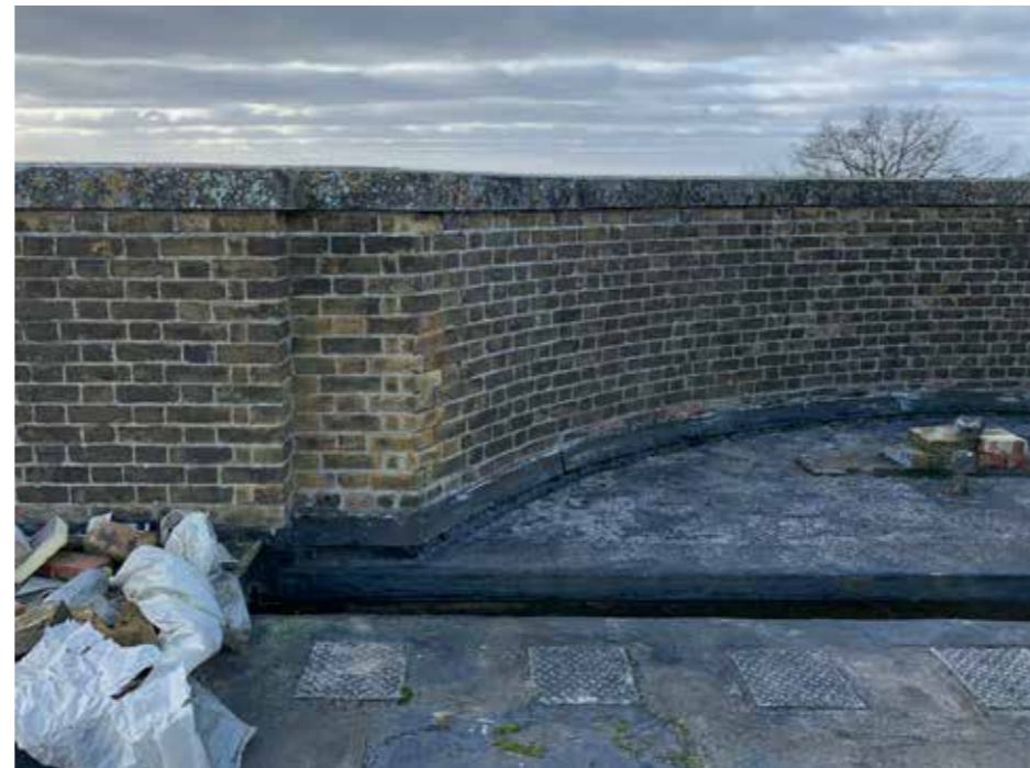
Plate : 27 South parapet wall to be rebuilt.
