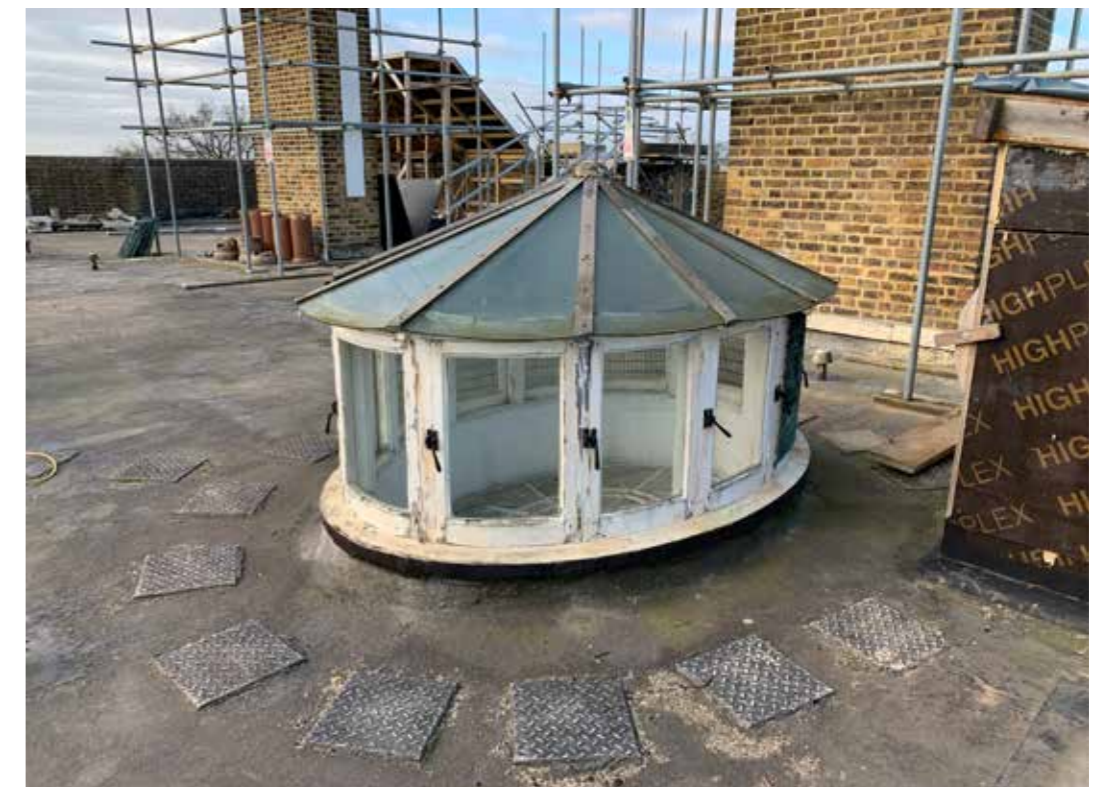
Plate : 50 North east roof lantern with modern top in poor condition. Consent has been granted for its replacement as described elsewhere.
