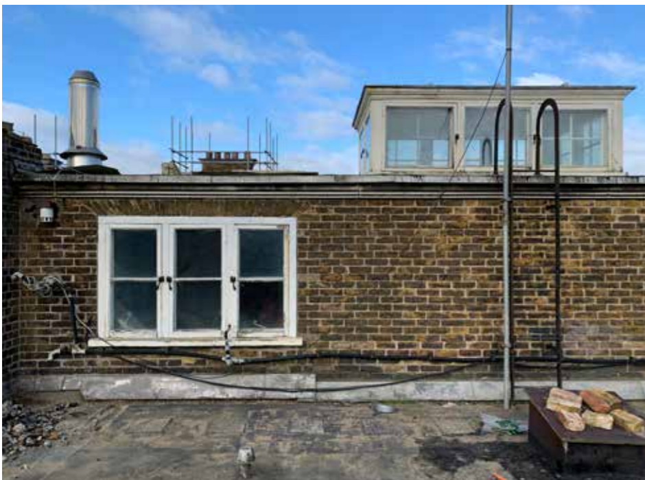
Plate : 44 Edwardian roof lantern and water tank room. Inadequate access to the roof lantern and the projecting boiler flue could be improved.
