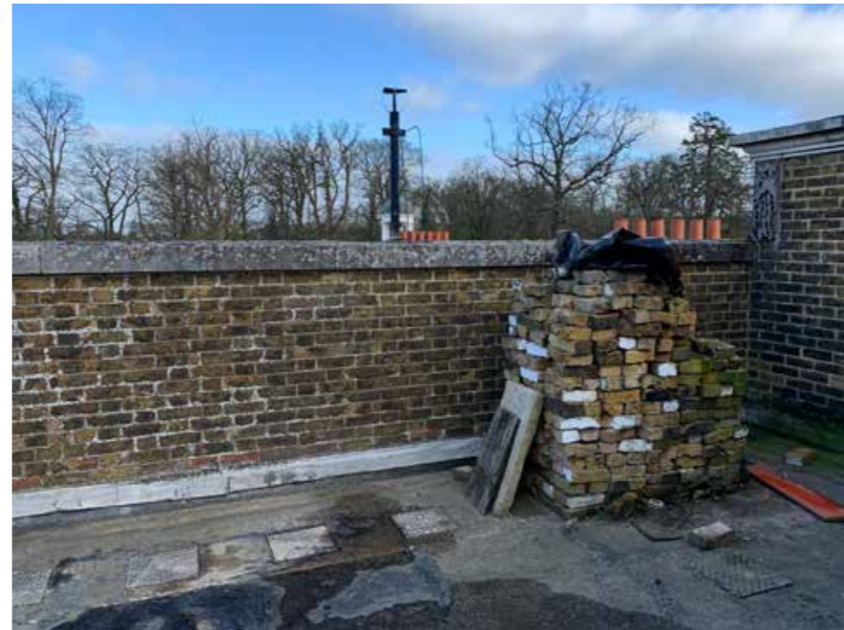
Plate : 12 Northern parapet. Consent is granted to rebuild as described elsewhere and raise the height to better suit the height of the enclosure around the back stair.
