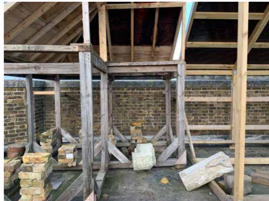
Plate : 24 North west corner of the parapet and a temporary mock-up of the roof form in timber to assess the pitch heights to ensure it complies with the consented drawings.
