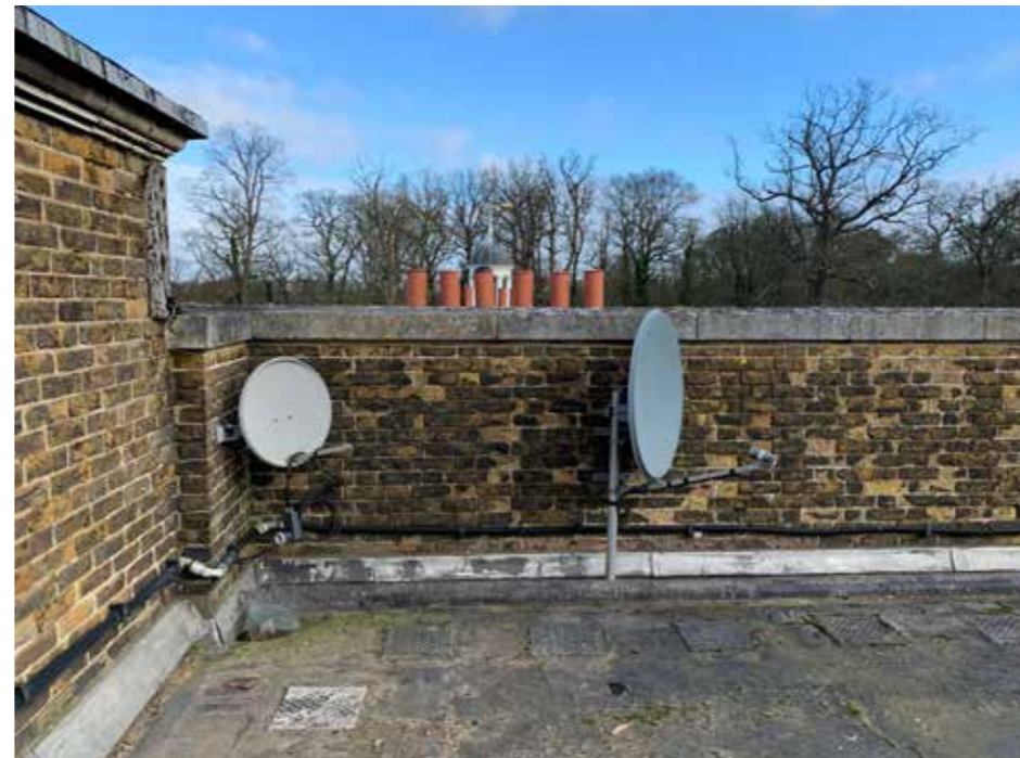
Plate : 42 North Parapet and satellite dishes (to be removed). Consent is granted to rebuild the parapet in a brick facing and tuck pointing to match the main house. The back stair block to the left has consent to be raised to accommodate the new roof.
