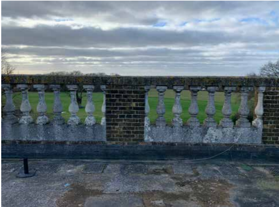
Plate : 29 Section of brick parapet on south facade showing bricks and pointing which do not match the main house.
