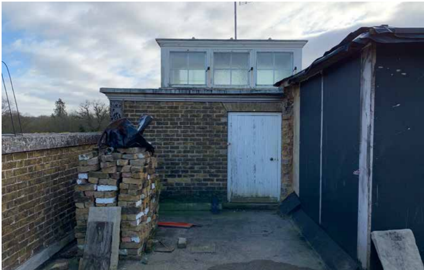
Plate 4: Below: Photograph of Edwardian Lantern taken in 2018. The consented roof clashes with this roof light and will need to be re-designed. The opaque glass and opening casements are more modern and there is little architectural merit in this element as a feature over the back stair on the rear elevation.
