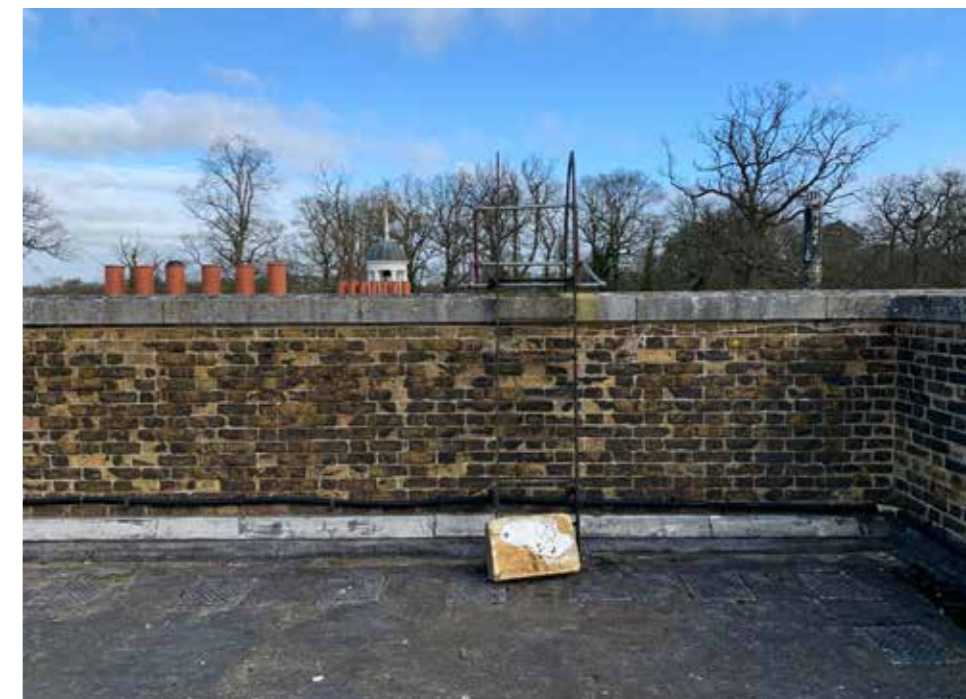
Plate : 40 North parapet and (dangerous) escape ladder. Consent has been granted to rebuild this parapet and provide an upgraded fire escape route to comply with Building Control.
