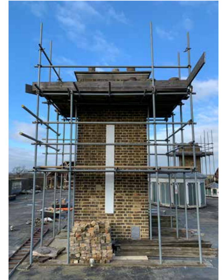
Plate :55 South-east Chimney stack to be raised above new consented roof and new Georgian pots to be added
