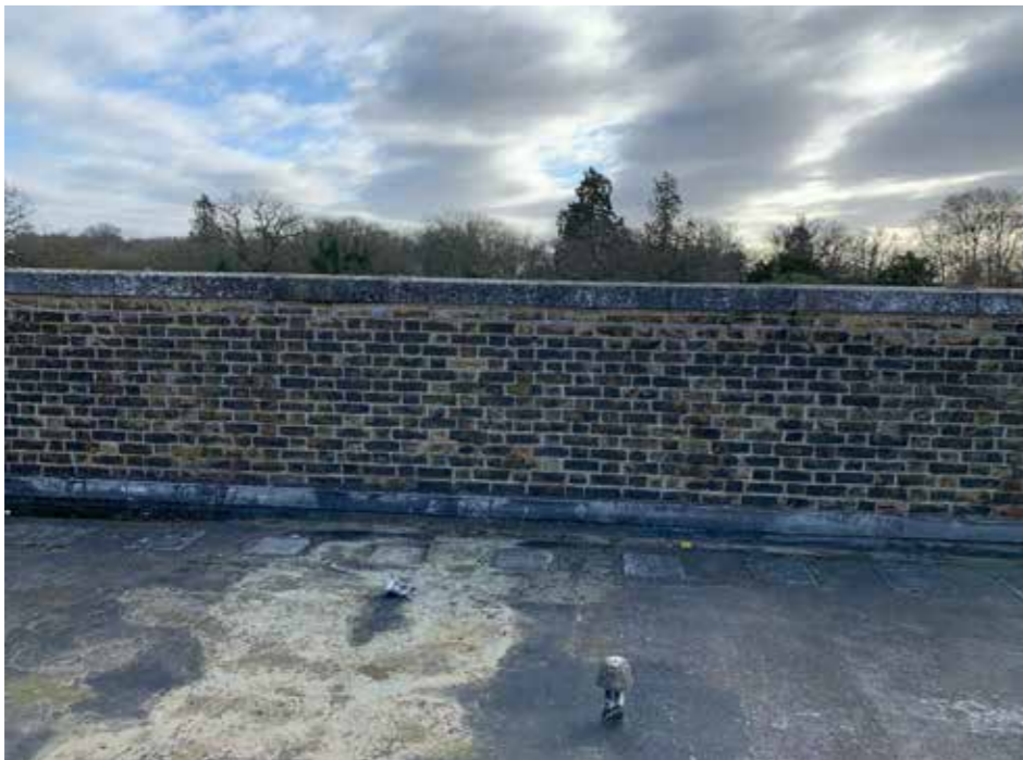
Plate : 38 Eastern parapet with brickwork and pointing which are of a much lower quality to the main house facing brick.
