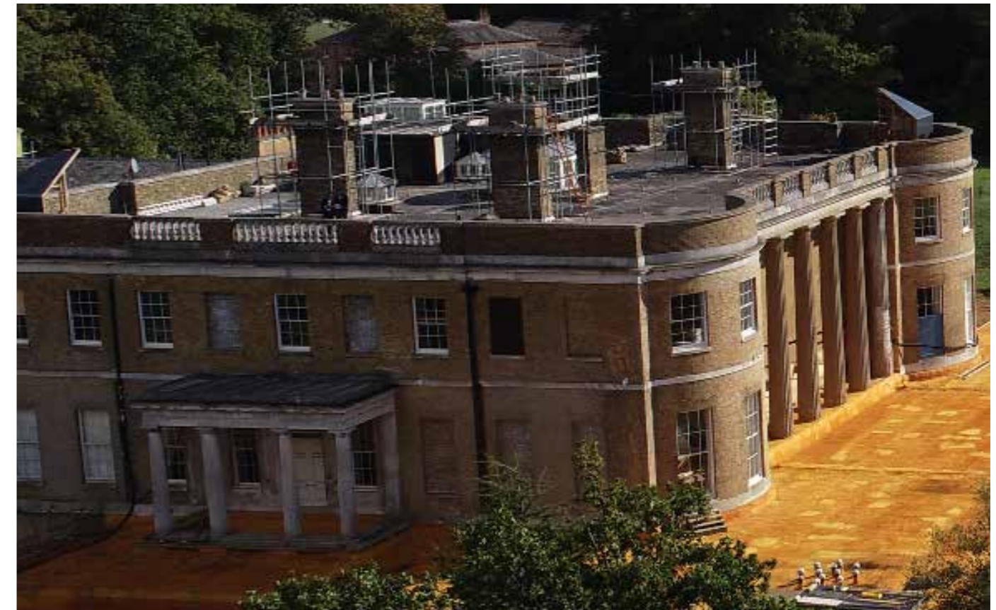
Plate 5: Below: Photograph of Sacombe House taken in 2018. Mock ups to show the height of the new roof can be seen at the corners. The Edwardian roof lantern can be seen in the background.
