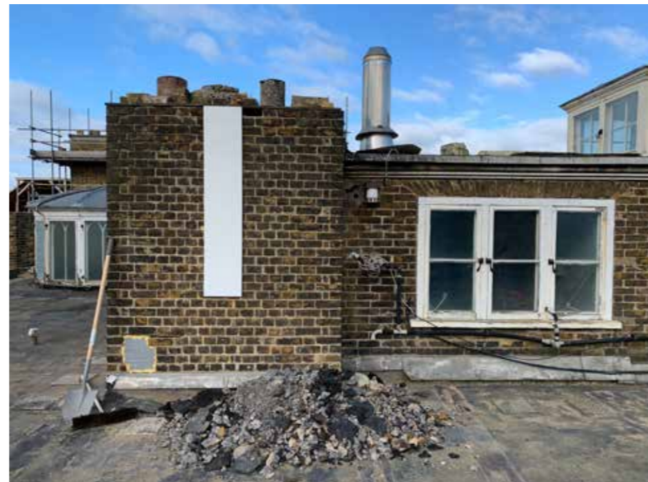
Plate : 45 North East Chimney stack and kitchen boiler flue. Casement window to water tank room has consent to be removed.
