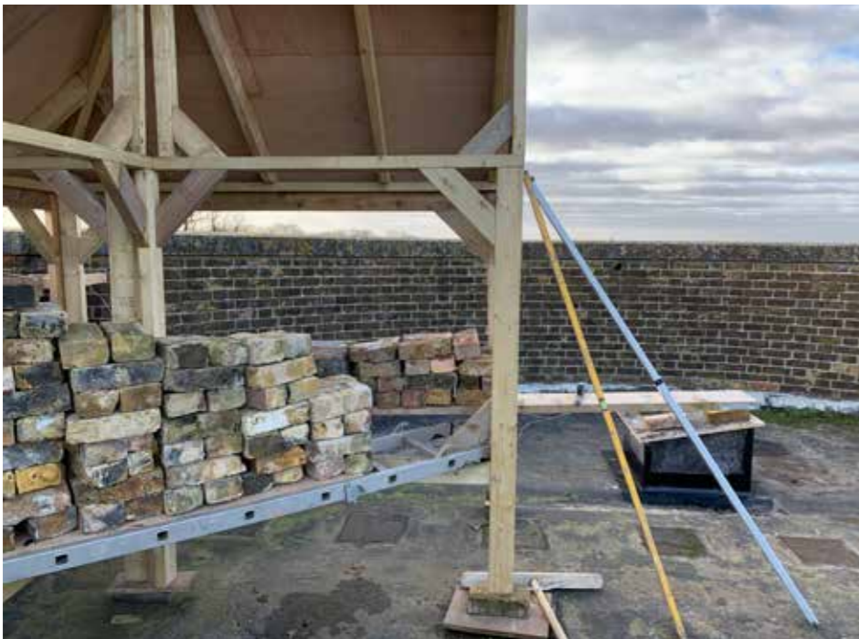
Plate : 32 South east parapet and curved bay forming terrace at roof level
