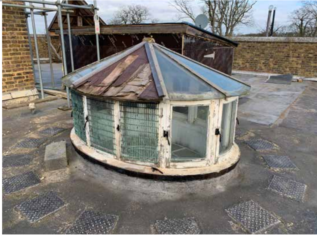
Plate :51 North west roof lantern with consent to be replaced with an oval 'walk-on glass. The underside and lay light is to be retained.
