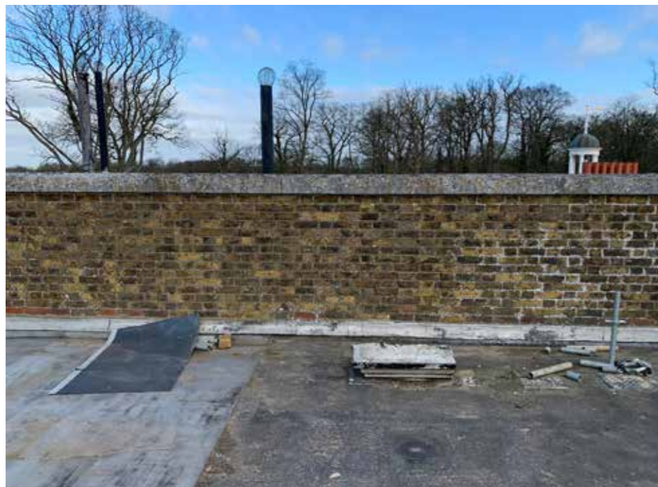
Plate : 14 Northern section of parapet and vent pipe. All service pipes have consent to be hidden or replaced in black cast iron. The parapet has consent to be rebuilt.
