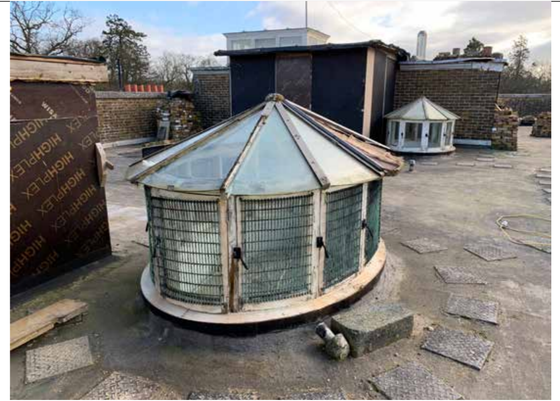
Plate :52 Both roof lanterns with consent to be replaced with oval 'walk-on glass. The underside and lay lights is to be retained.
