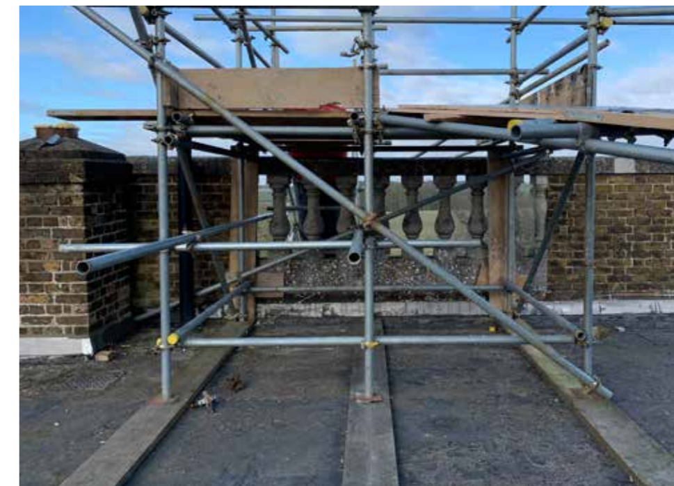
Plate : 22 Western parapet and mini chimney stack serving the Study on the Ground Floor. Consent is granted to rebuild the parapet and incorporate this flue into the wall to comply with Building Control.
