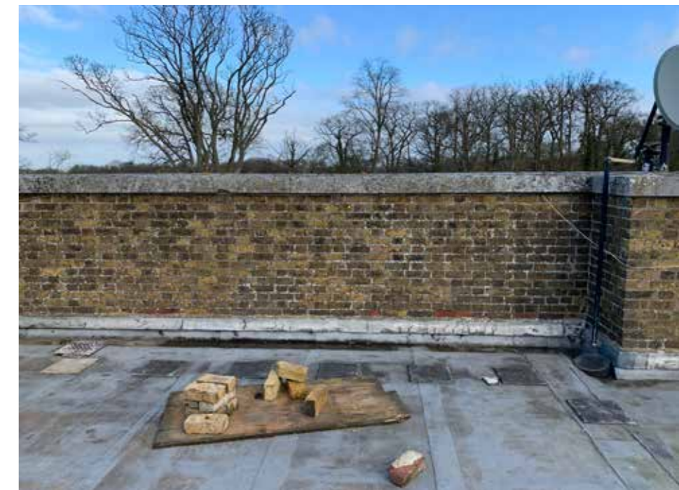
Plate : 16 North west section of Parapet. Consent already given to rebuild in brickwork and pointing to match the main house with sections replaced with stone bottle balusters to match the existing.
