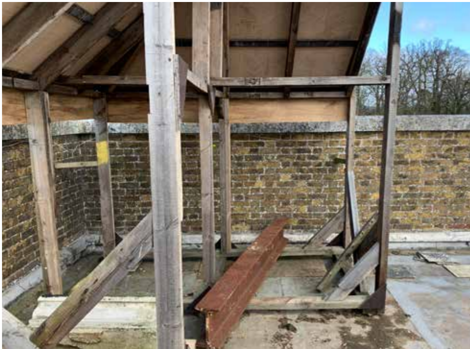
Plate : 17 North west corner of the parapet showing part of the mock-up for the new roof to establish the correct pitch and heights.
