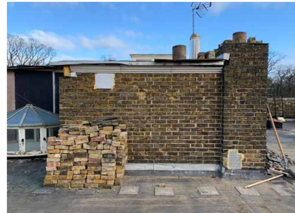
Plate : 46 North East Chimney stack which is far too low for the consented roof. The wall here is partly consented to be removed and is constructed in concrete block and brick facing with cavity insulation.
