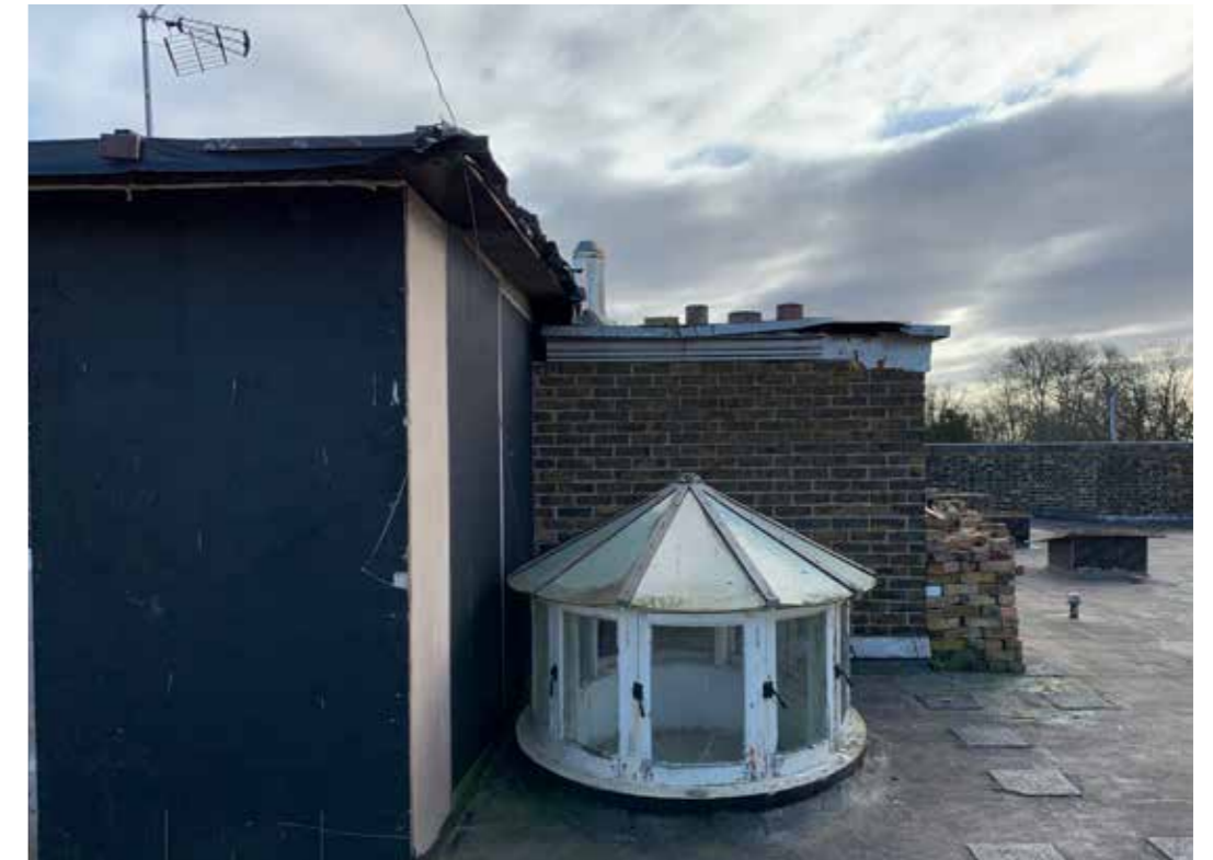
Plate : 48 Service lift shaft and lantern in poor condition has consent to be replaced with an oval 'walk-on glass. The underside and lay light is to be retained.
