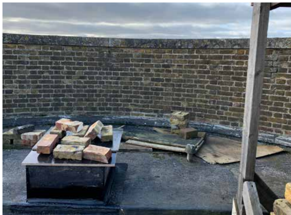
Plate : 26 Curved Parapet over the south west bay. The proposals seek to make use of this existing terrace accessed through the opening section of the roof.
