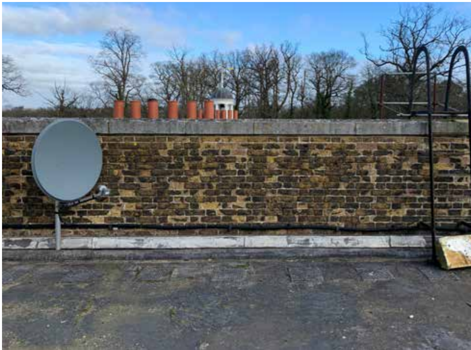
Plate : 41 North parapet and existing escape ladder. Consent has been granted to rebuild the parapet with new stone bottle balusters to match the existing. Additional escape has been requested from Building Control in the event of a fire.
