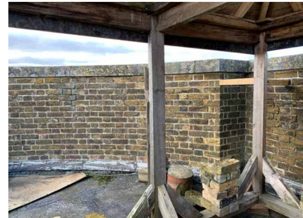
Plate : 25 South east corner of the parapet over the bay window in the Study. Consent has been granted to rebuild this in facing brickwork and pointing to match the main house disburshed with stone bottle balusters to match the existing over the windows below.
