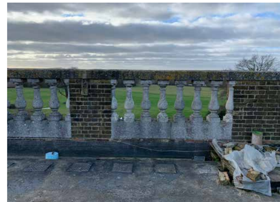
Plate : 28 Example of the existing stone bottle balusters on the southern section of the parapet inserted over the windows below.
