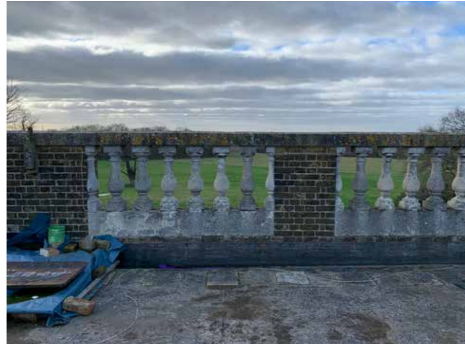
Plate : 30 South Parapet and existing bottle balusters to be retained and copied for areas where new balusters are to be inserted.
