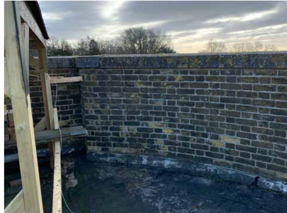
Plate : 33 Poor brickwork and pointing to the back of the parapet on the bays to be replaced with brickwork and pointing to match the main house with stone balusters over windows below.
