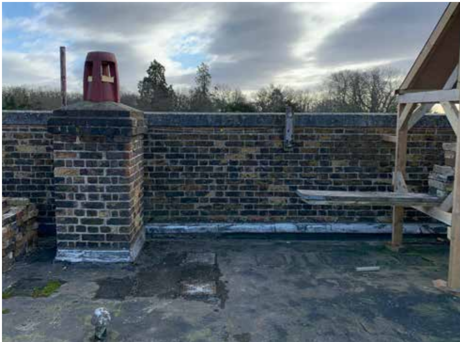
Plate : 35 Eastern Parapet and mini chimney stack serving the Drawing Room on the Ground Floor. Consent is granted to rebuild the parapet with stone bottle balusters and incorporate this flue into the wall to comply with Building Control.
