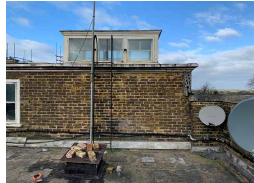
Plate : 43 Edwardian roof lantern over the back stair has consent to be removed and the walls raised to accommodate the new roof.
