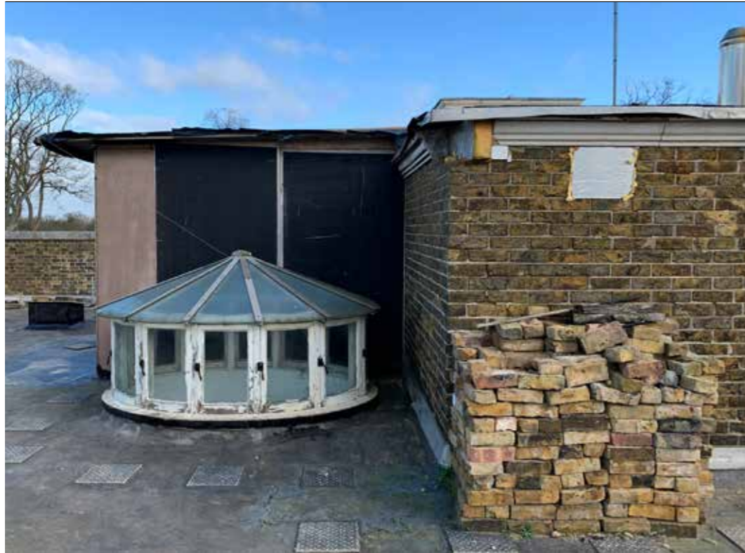
Plate : 47 Roof Lantern, water tank room and service lift shaft. Consent for the brickwork, concrete block and concrete lid to be replaced. The stone cornice is to be retained for reuse on the chimneys to supplement the existing.
