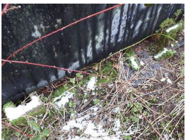
Surface-mounted oil storage tank. No evidence of leaks at base
