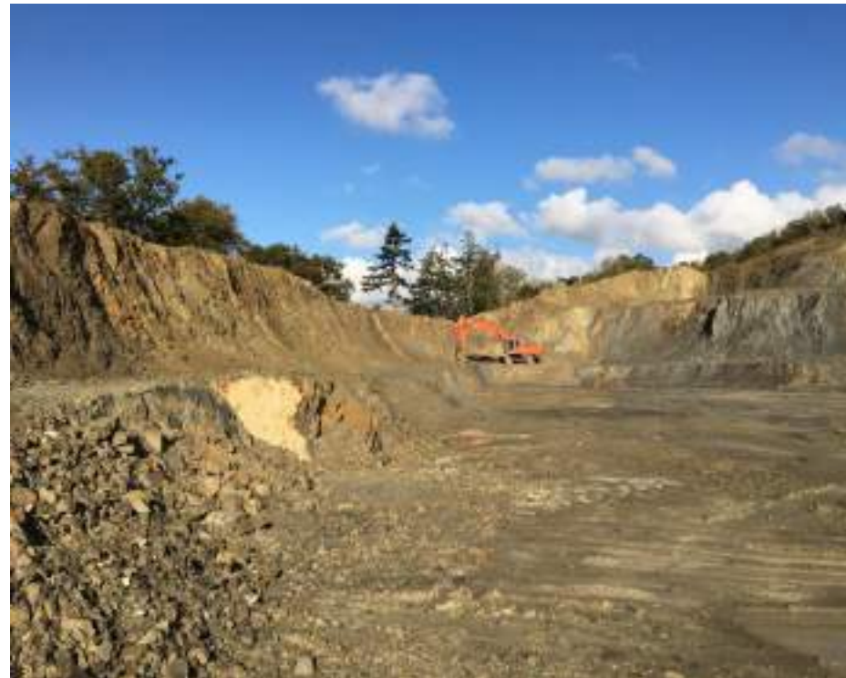
Photograph 7: General view looking north along the western excavation. Some spalling at base of slope but excavation appears stable at 70-80°.
