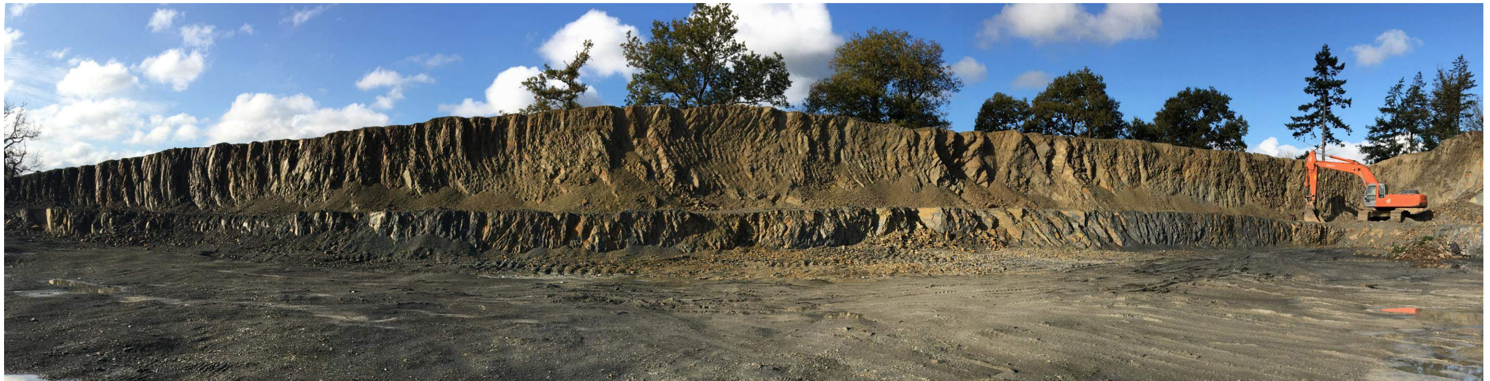
Photograph 5: Panoramic view of western excavation face showing 1.5m high lower face and 2-4m high upper face. Some minor spalling present but no signs of significant instability. Angle of face is variable up to approximately 70-80°. Face is dry with no indications of groundwater seepage.
