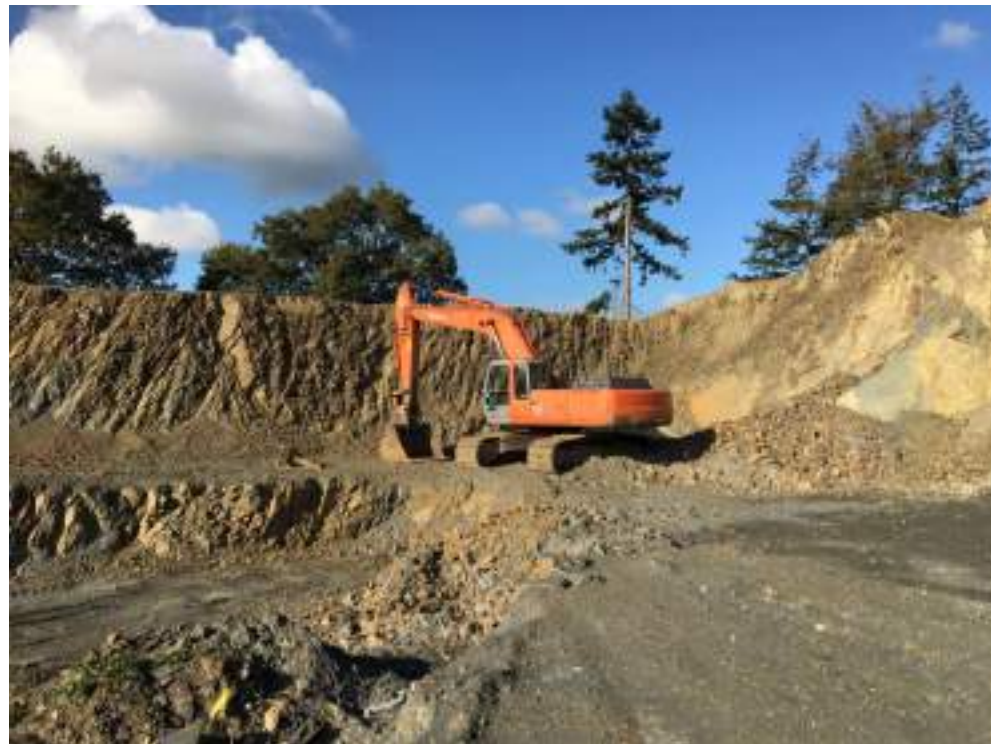
Photograph 2: View looking north into corner of existing excavation adjacent to new access road.
