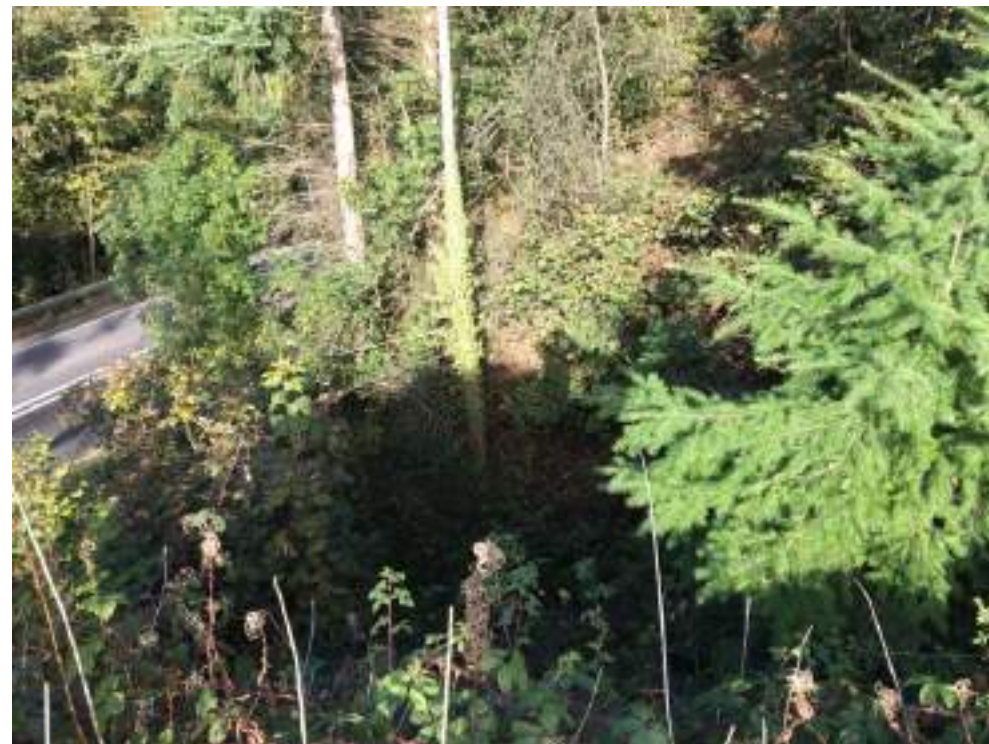
Photograph 12: View looking down into former highways cutting with 50-60° vegetated slopes. No indications of tension cracking or instability although some historical spalling evident at base of slope.
