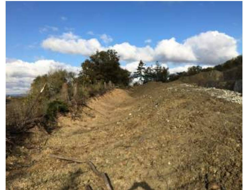
Photograph 8: View looking northern along crest of western excavation. Vegetation has been cleared with good exposure. No indications of tension cracking, deformation or signs of instability.
