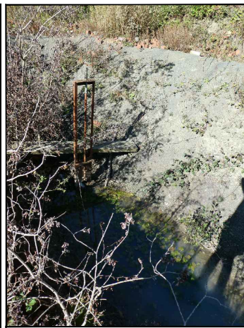
2. Site drain with penstock flow control
