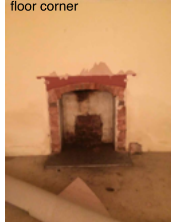
Fire surround torn off in Siting Room 1
