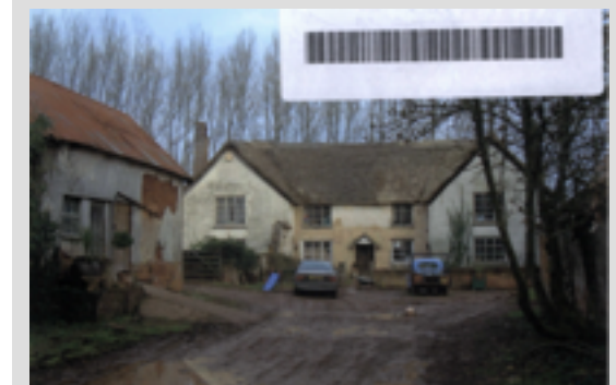
Photos of Great Barton submitted with application 02/P0519 illustrating building condition at that time.
