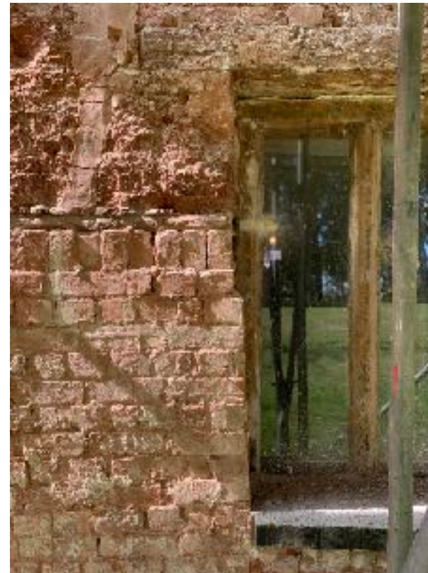
Previous: 4 light window frame with 20C panes inserted. Bottom rail of frame submerged by cast inset cill
