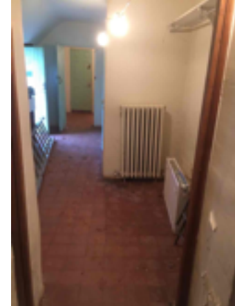
View of Utility in Out Shut
