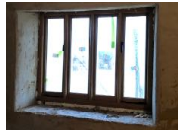
Now: New four light oak framed window and cill installed. Historic frame retained on site.
