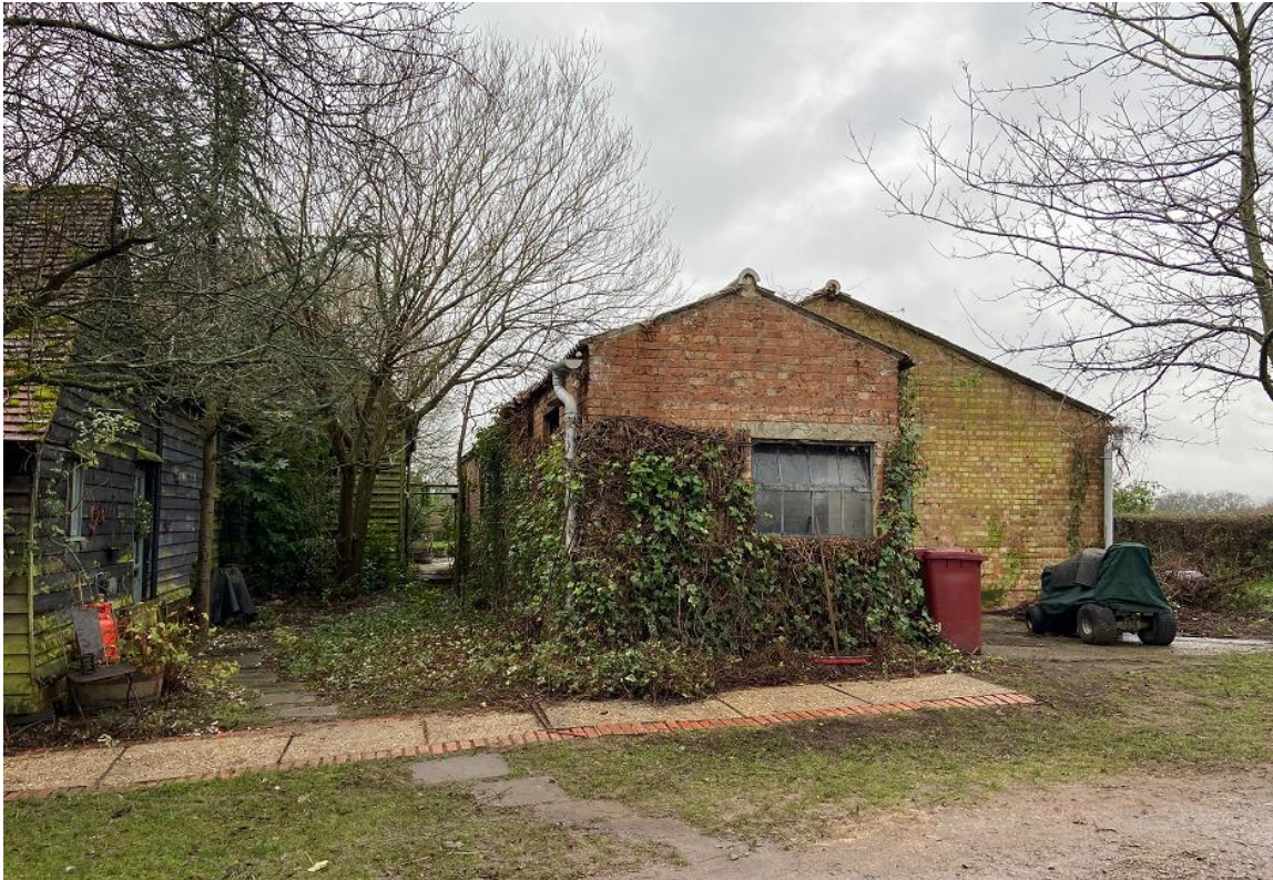
Figure 9 : A view of the cowshed from the east, with the barn and additions to the left
