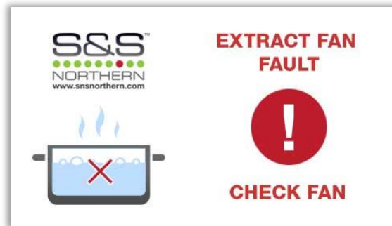
Fig.3.9 Extract fan fault display screen.
