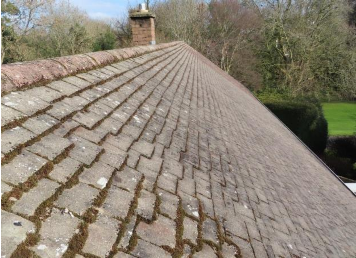
Photograph 6. View of part of the south elevation roof-slope of Section A. Looking east from west.
