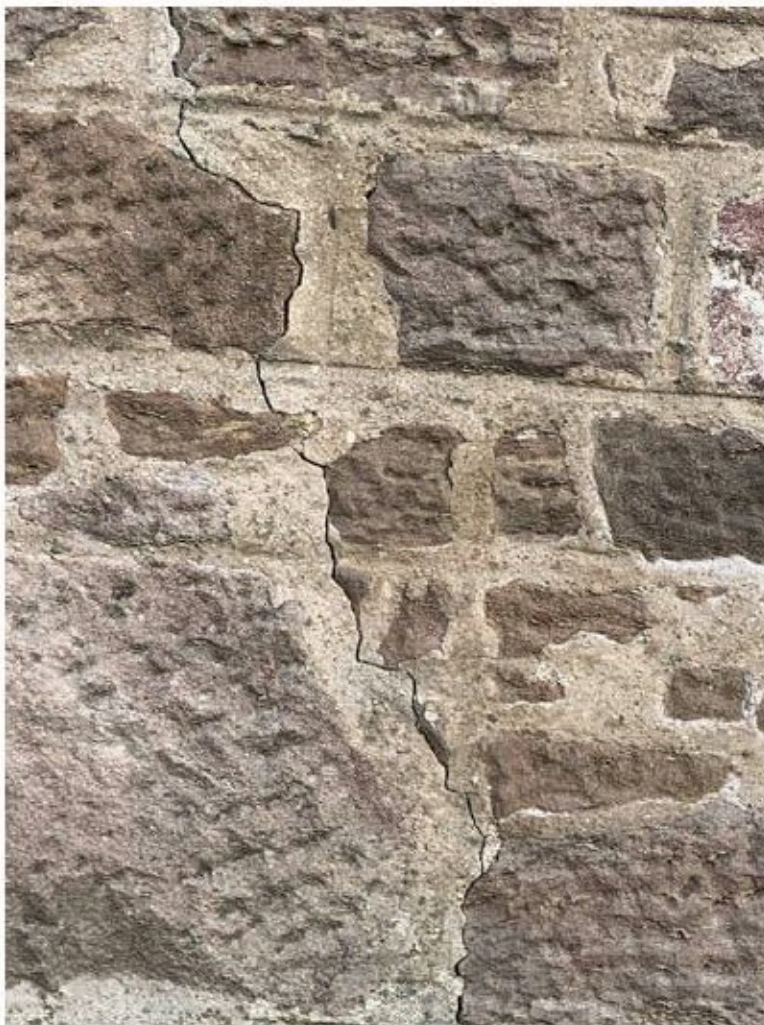
Figure 10: North East Elevation – Typical Crack
