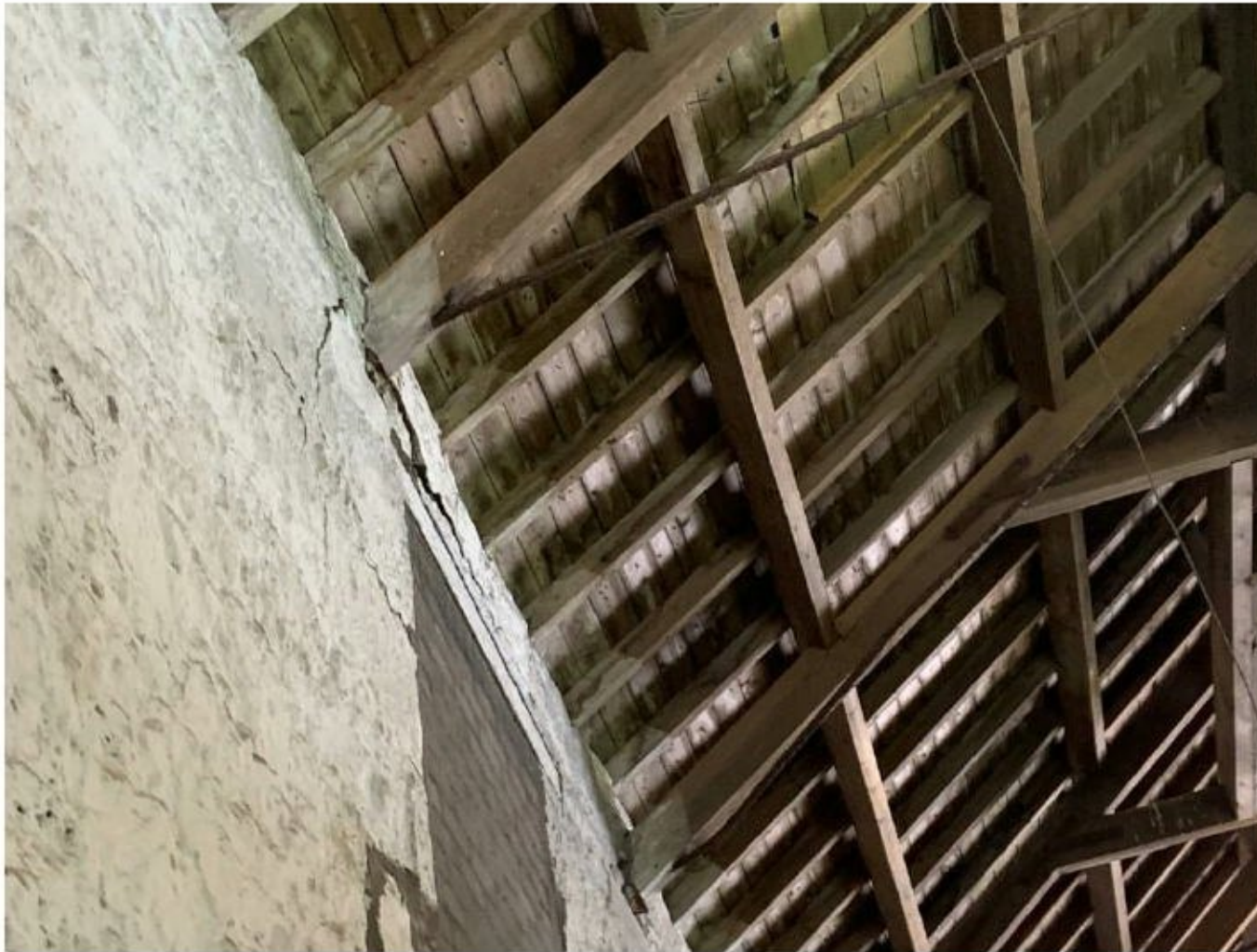
Figure 19: Internal North East Elevation –Wall Leam, Wall Displacement, Patches & Cracking
