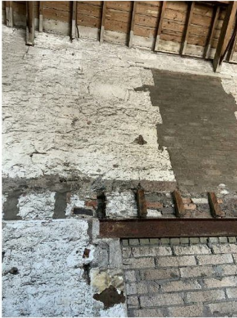
Figure 21: Internal North East Elevation –Intermediate Floor, Patches & Cracking
