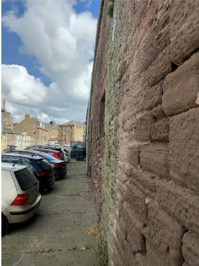
Figure 5: North West Elevation – Wall Lean
