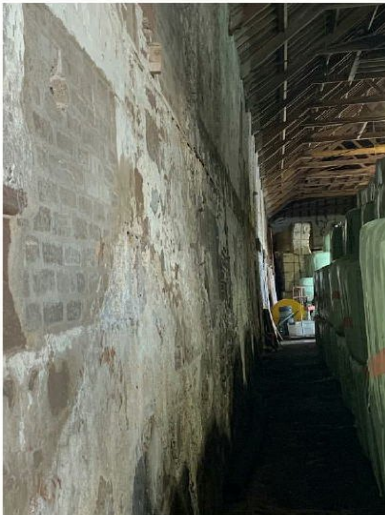
Figure 16: Internal North East Elevation –Wall Lean, Weathered Stone, Patches & Cracking
