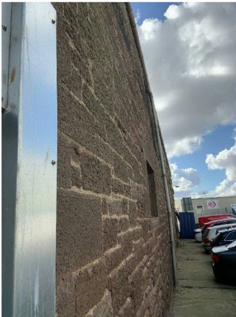
Figure 6: North West Elevation – Wall Lean
