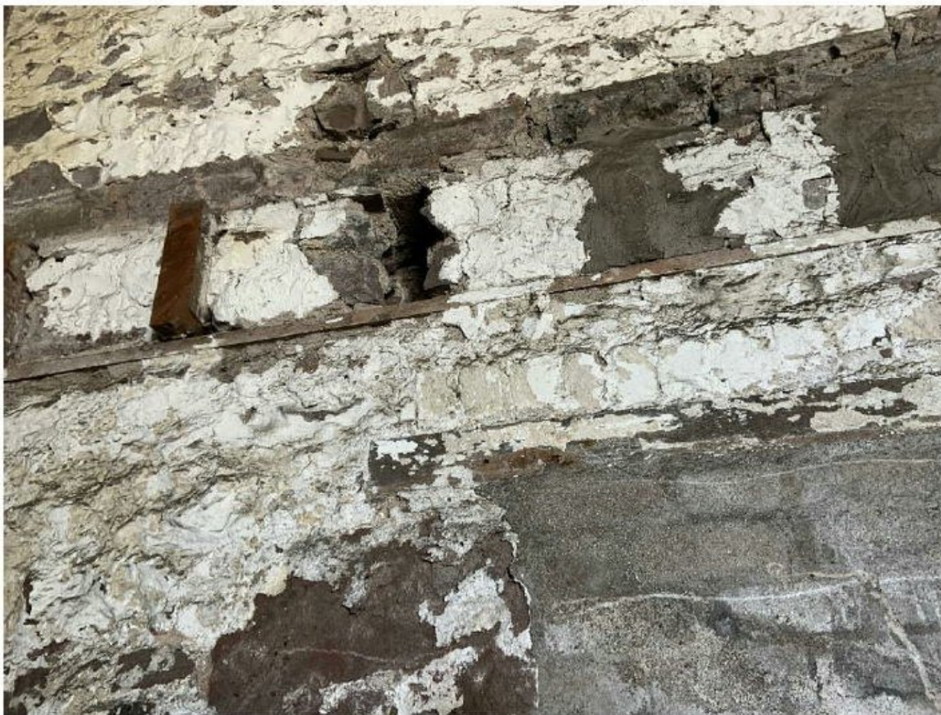
Figure 22: Internal North East Elevation –Intermediate Floor, Patches & Cracking
