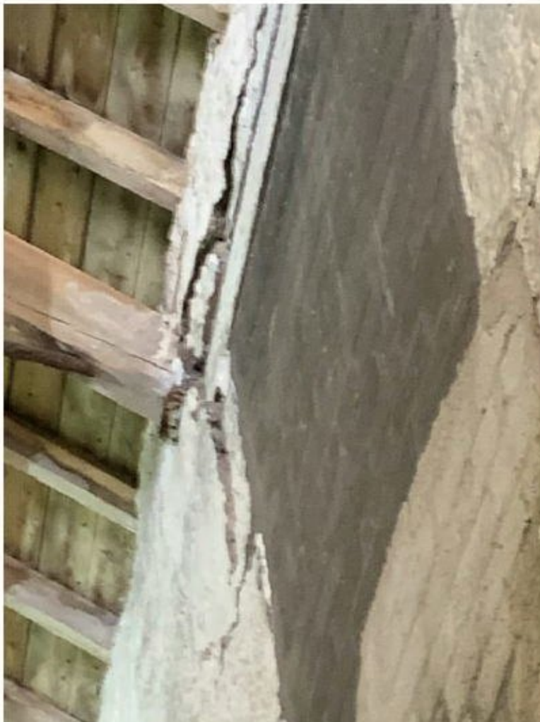
Figure 18: Internal North East Elevation –Wall Leam, Wall Displacement, Patches & Cracking
