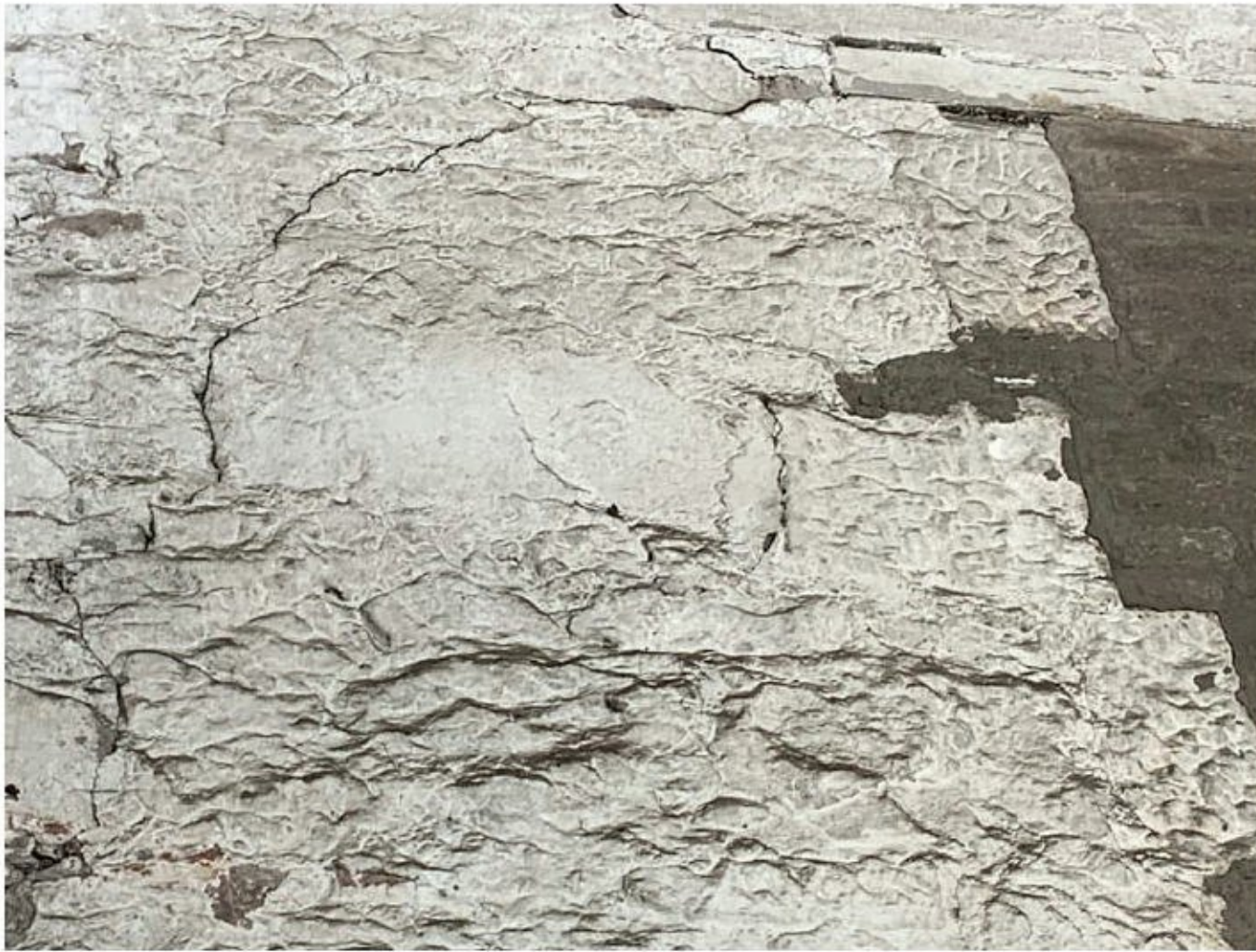
Figure 23: Internal North East Elevation –Diagonal Crack
