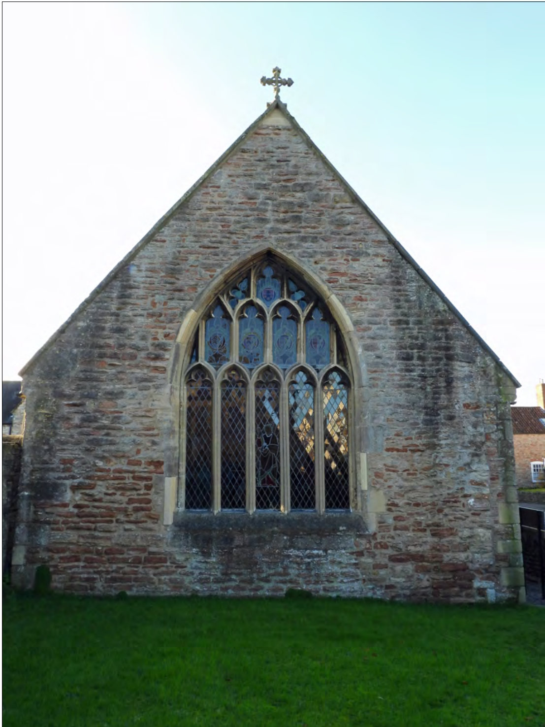
The East wall of the Chapel - the north-eastern quoin has been rebuilt - note the modern insertions around the window showing as paler blocks.
