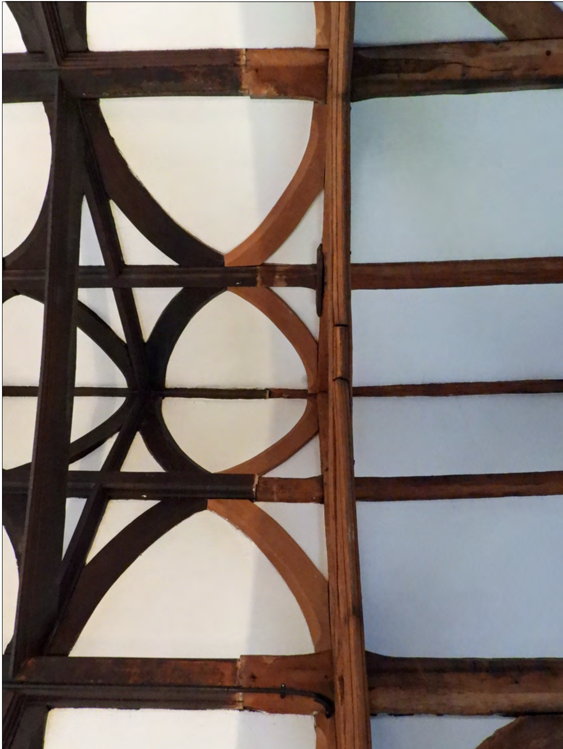
Repairs following the removal of the 1850 cross wall dividing the chapel from the accommodation to the west, showing as paler timber.
