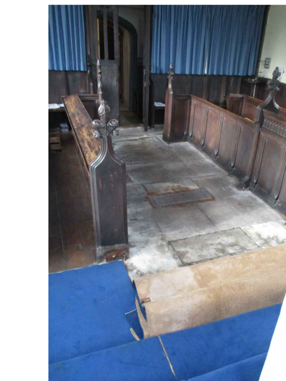
The carpet pulled back in the central aisle revealing a worn but not archaeologically significant limestone floor. The good quality priests stall is on the north side.
