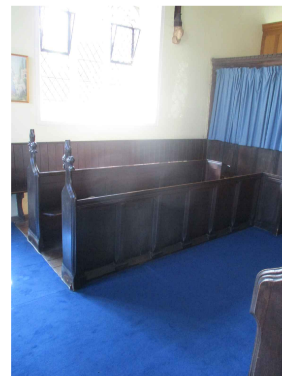
The existing benches and carpeted floor over a combination of a stone and suspended timber floor. There is no cross ventilation.
