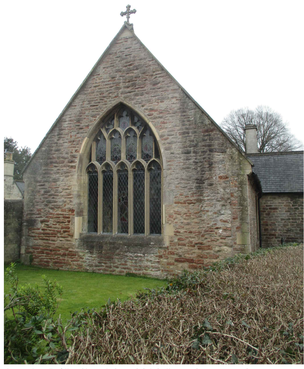
The East Wall of the Chapel. Open joints in the copings are causing water to flow into the wall. High ground levels are the cause of plaster problems internally.
