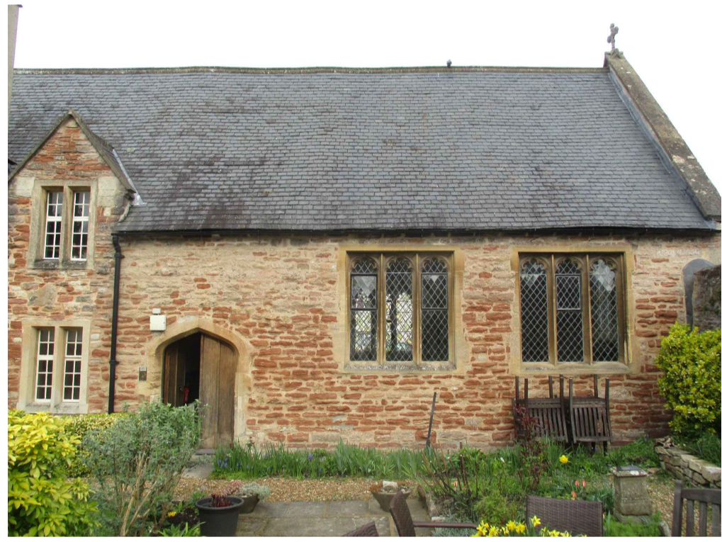
The South Wall of the Chapel. Cement pointing should be removed and ideally the wall should be repointed. The ground gutter in front requires repair.
