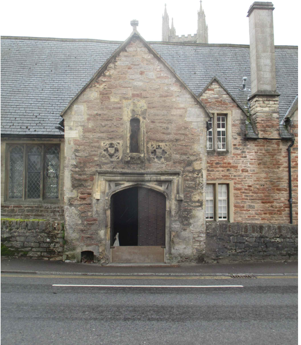
The North Porch almshouse entrance. The stonework condition is poor and the entrance poorly defined. Cement mortars are also present.
