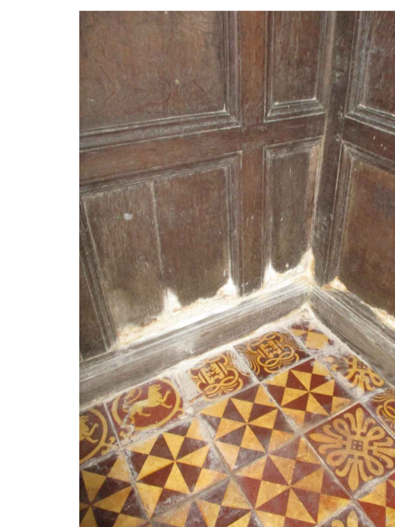
Decay to Sanctuary panelling in part caused by high ground levels outside.
