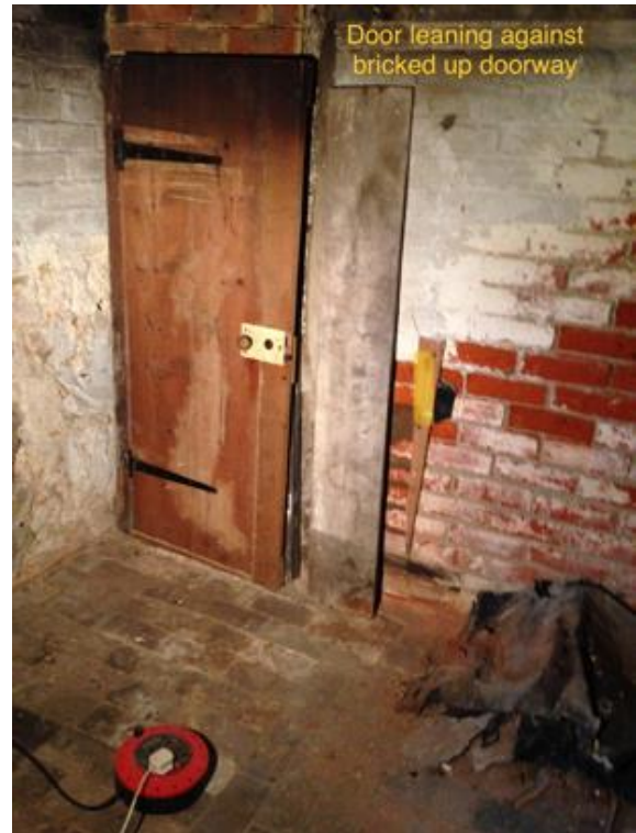
Former door leaning up against bricked up door our side
