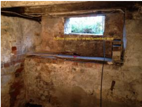
This photo shows the opening to street level through which access has been gained..
