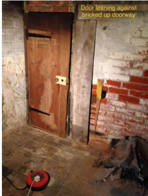
Our side (no 37) Door is bricked in and unattached
