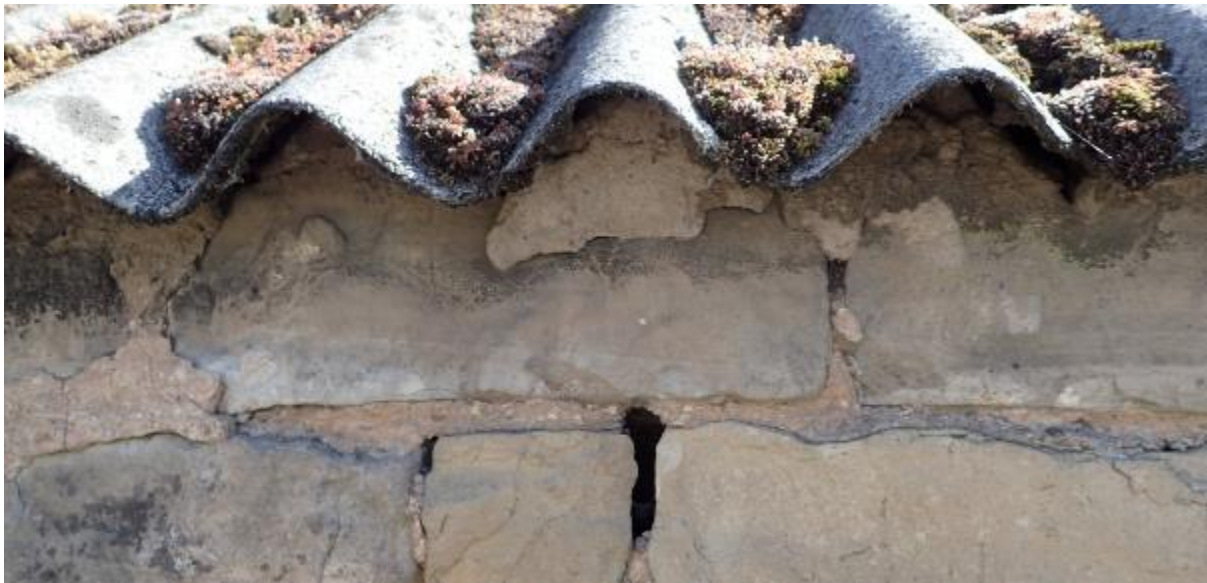
Photograph 8: An example of gap in stonework at west elevation
