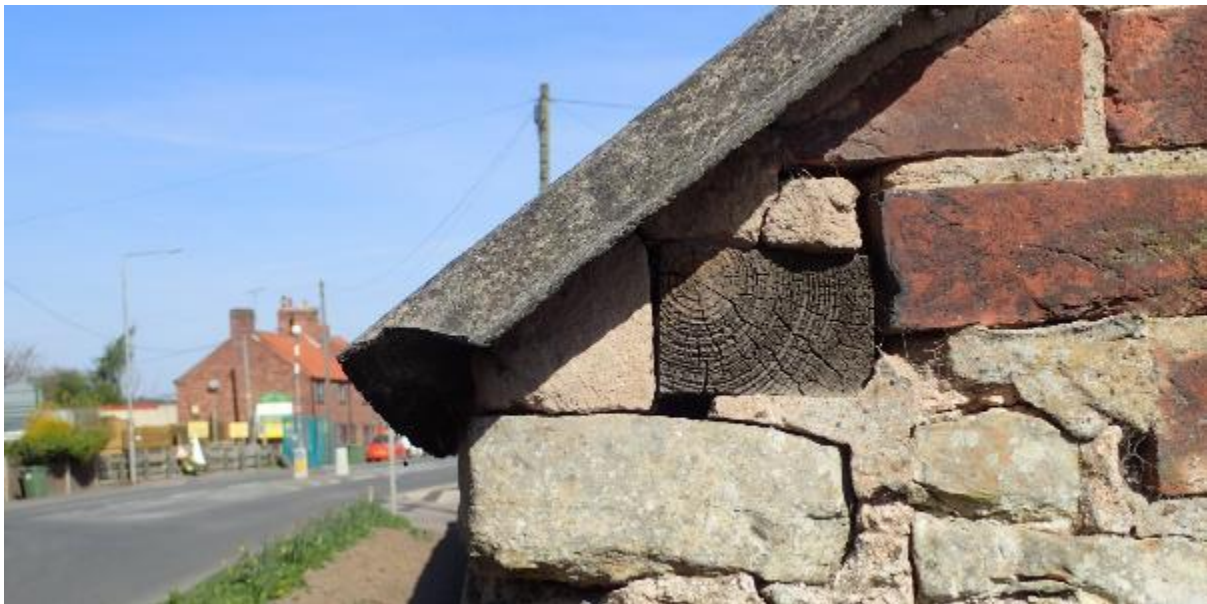
Photograph 6: Gaps around wall plate at south elevation
