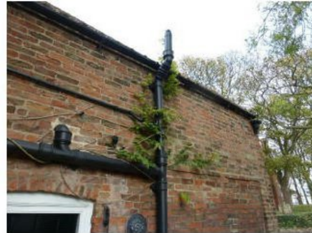
Existing SVP for potential new en-suite drainage
