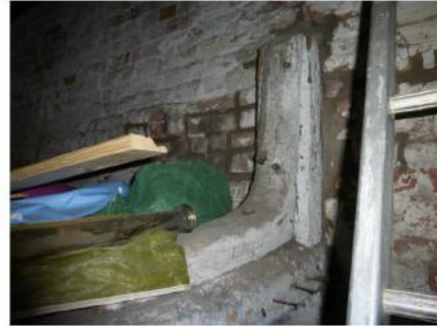
Blacksmiths Forge existing first floor beam to be retained Unusual, inverted knee brace to beam ends
