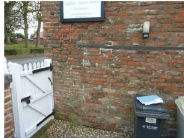
Blacksmiths Forge. Main entrance opening to be re-established.
