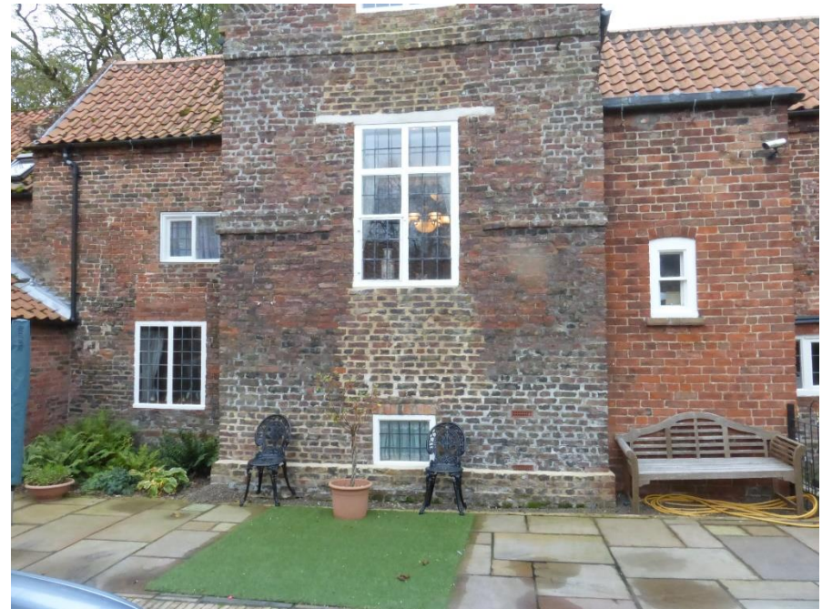
Existing window to the main staircase providing both design and scale elements for the proposed bedroom window. The design of the window reflects the eclectic mix of window styles found in the building over centuries of development and alterations. A Yorkshire sliding sash is also illustrated to the left of the main window at first floor.
