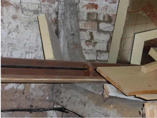
Blacksmiths Forge interior. Mezzanine position Unusual, inverted knee brace to beam ends
