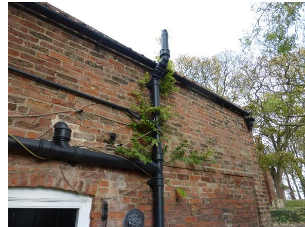
Existing SVP for potential new en-suite drainage
