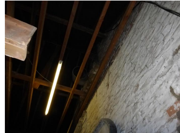
Blacksmiths Forge. Remains of flue from forge range
