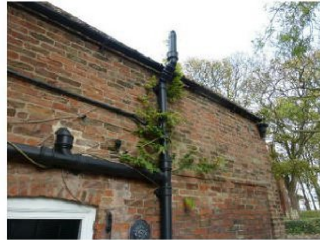
Existing SVP for potential new en-suite drainage
