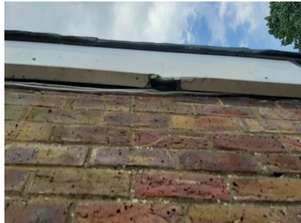
Plate 4.3: Gap in Fascia Board
