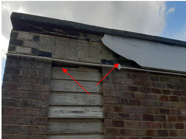
Plate 4.2: Gaps Above Doorframe and Between Fascia Board and External Brickwork
