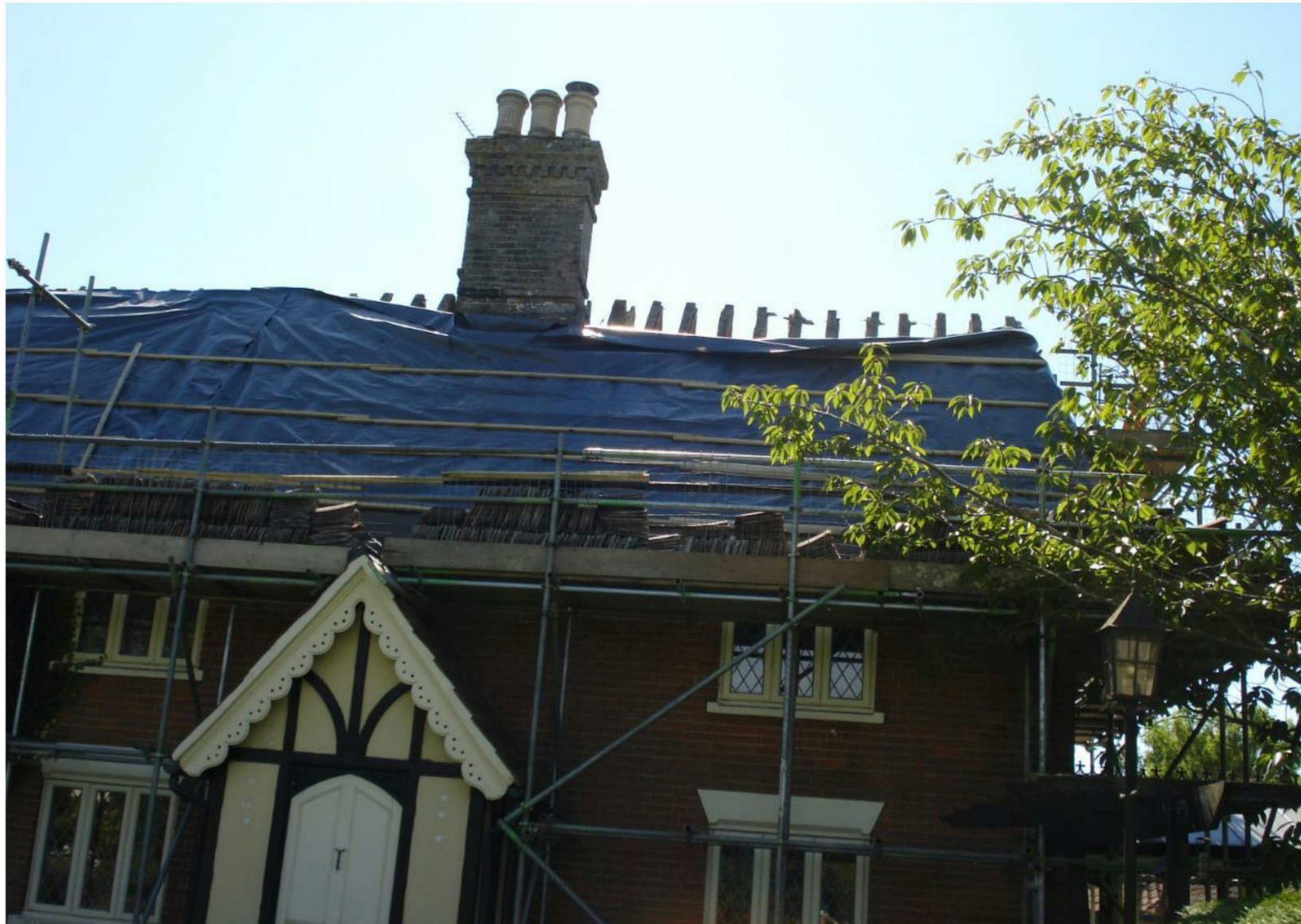
Photographs of the main house and annexe during the renovation works in 2014
