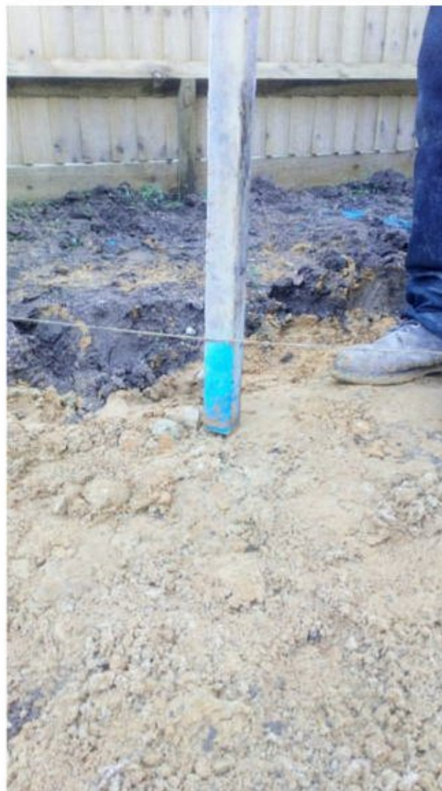
Placement of subsoil in plot and string lining to ensure correct depth in Plot 177
