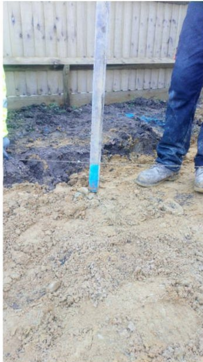
Placement of subsoil in plot and string lining to ensure correct depth in Plot 177
