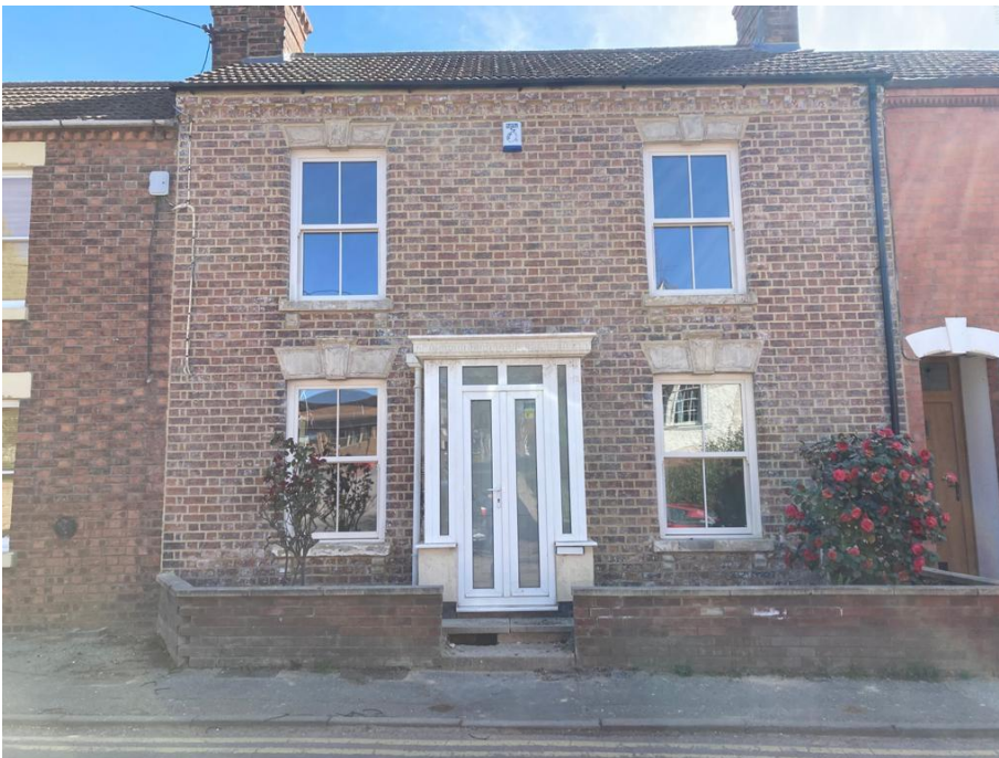
Photo of front elevation with render removed.
