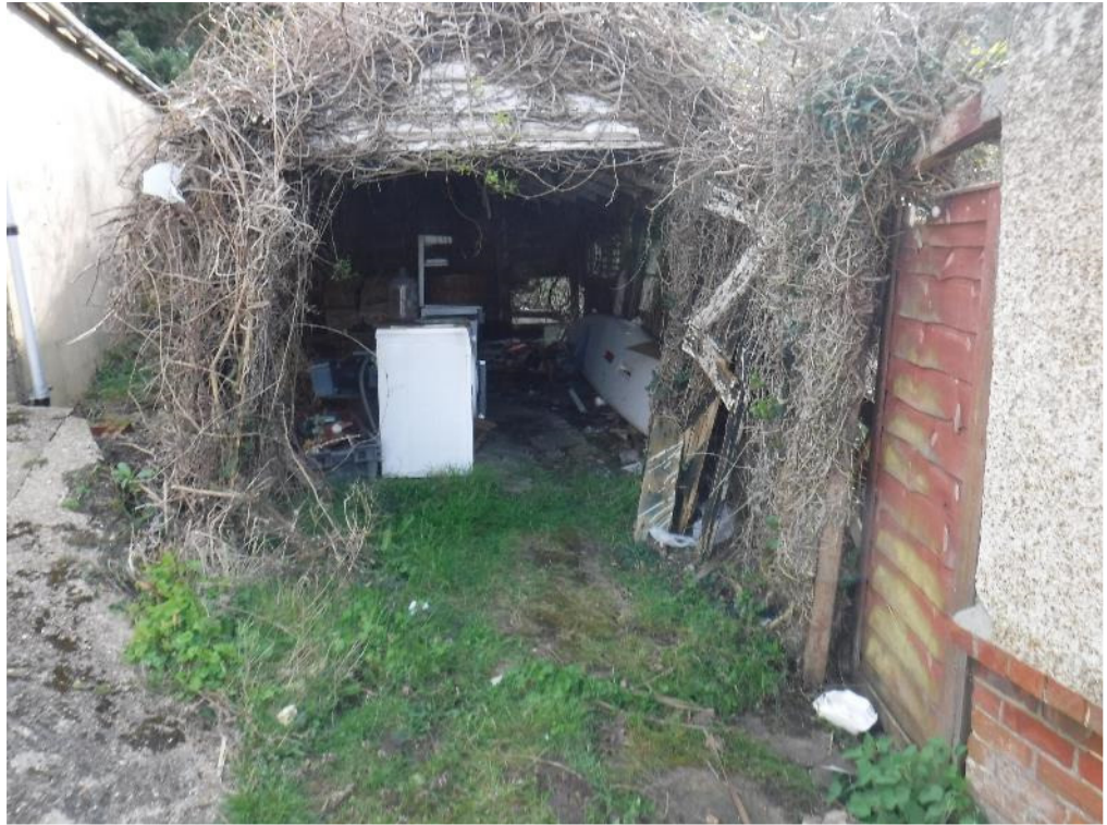
Dilapidated garage at northeast
