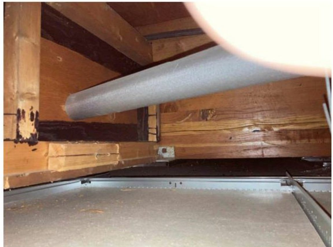
Figure 5 - Roof structure over the kitchen, with a combination of simple joists, timber I-sections and Glulam members.
