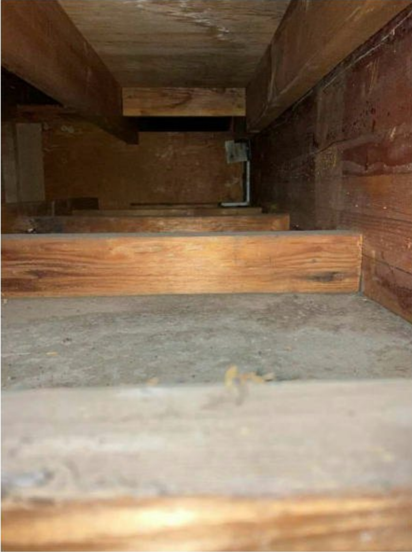
Figure 4 - Construction over the main hall, with primary Glulam members supporting two layers of timber joists, secondary composite I-sections are also visible here.
