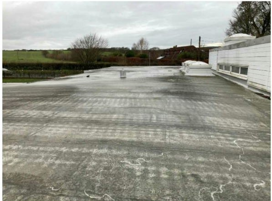
Figure 3 - Roof surface, showing deviations capable of accumulating some ponding, as well as the higher level roof which may result in snow drift loading against it. The shallow roof pitch and negligible gutter gradient are also visible here.
