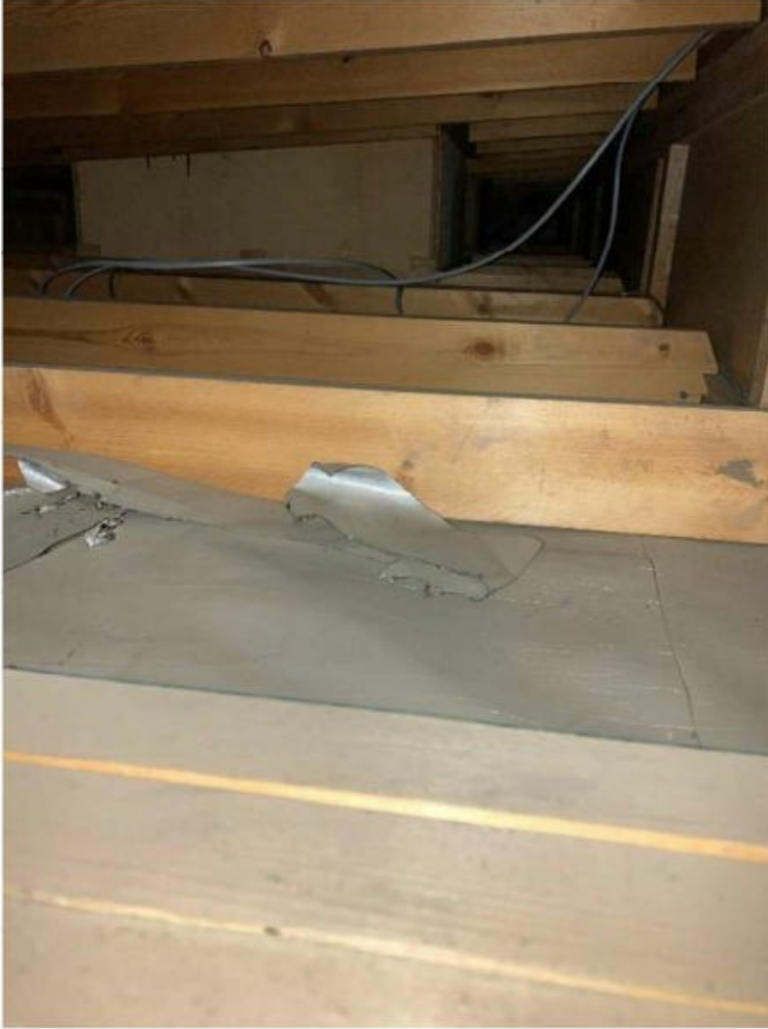
Figure 2 - Roof construction over the western classrooms, showing primary compound I-section joists with two layers of secondary joists.
